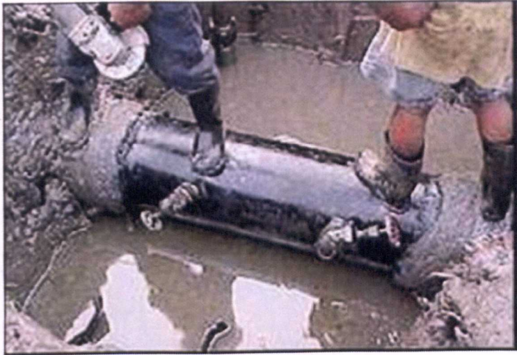
Figure 6.10: Illegally Installed Valves to steal Oil from Pipeline System
