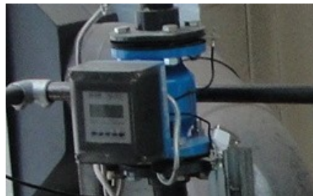
Figure 4.7 Electromagnetic Flow meter within vertical test section
