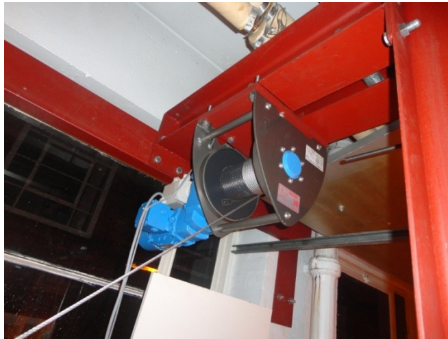
Figure 6.8 Actual photo of the electric wire rope winch
