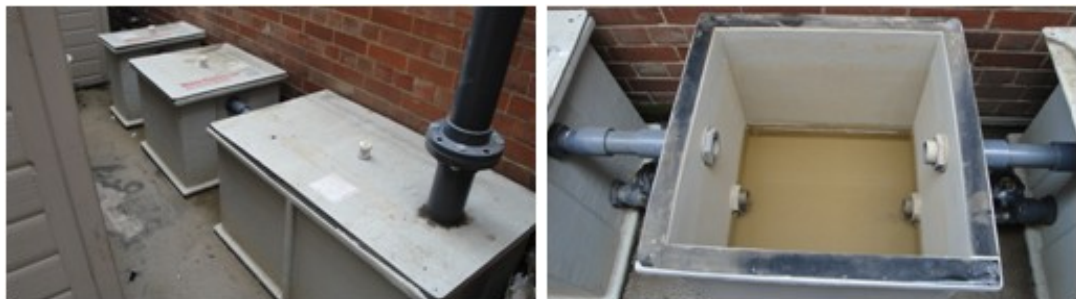
Figure 6.25 Actual photograph of the drainage system
