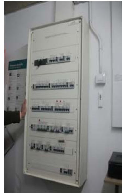
Fig.6.49. M:FP 0.0 P:23 Electricity box
