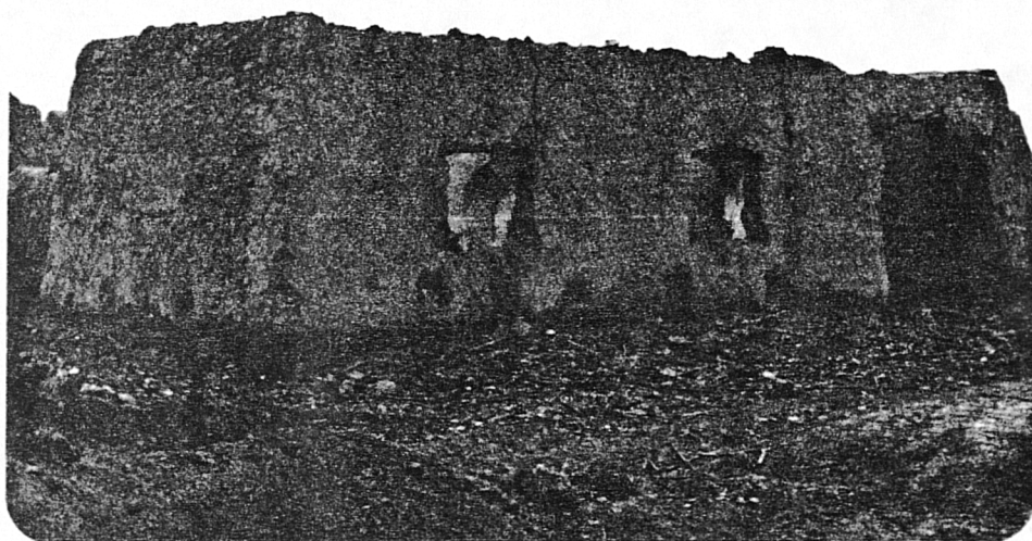
Plate 1-3: The effect of rising damp on mud built walls
