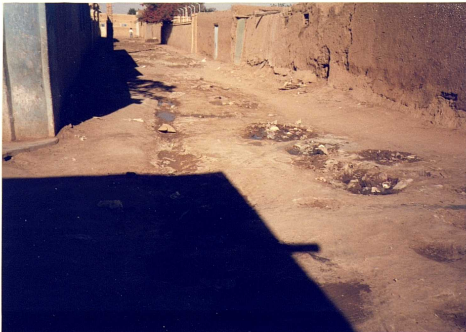
PLATE (6.4): Roses and Pot-holes on a littered narrow street, the contractions of Al-Busta Ganoub.
