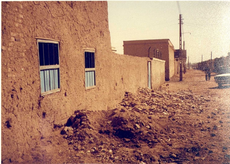
PLATE (6.14): A main street on the southern side of Al-Umda Sharque. The leftover building materials on the left side represent the poor control and maintenance of such as a public property. Note, the height of the boundary wall and the two-level type windows that benefit residents from being overlooked by passers-by. Also, note the only thing added to the street were the electricity poles.
