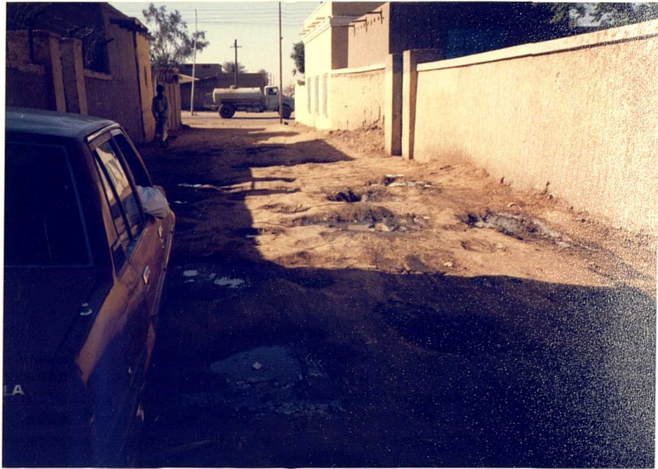
PLATE (6.3): Many of Al-Busta Ganoub streets were full of pot-holes trapping rotten water, especially during the rainy season, a situation that was neither safe for people nor for cars. (Note the tree-less/street shaded by the dwellings along its left side. Also, the neat dwellings to the right of the picture and the rough street, assentuting the difference between the private and the public domains.
