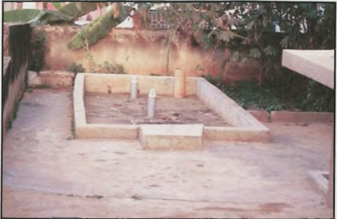
Plate 10 A typical household septic tank at the end of the drive way with vent pipes showing
