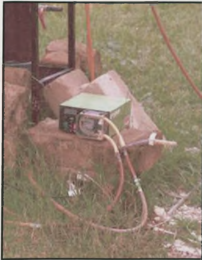
Plate 31 A WATSON MARLOW 505S Peristaltic Pump used in pumping the influent
