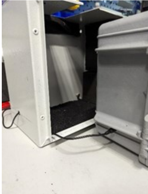
Figure 23: Connecting power cable to the sampler
