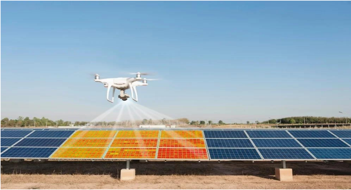
Figure 9. Thermal inspection of PV modules performed using an aerial drone equipped with an infrared camera [64].
