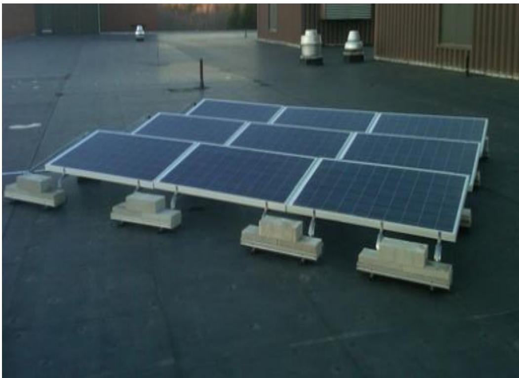
Figure 37. Examined PV system on the site [110].
