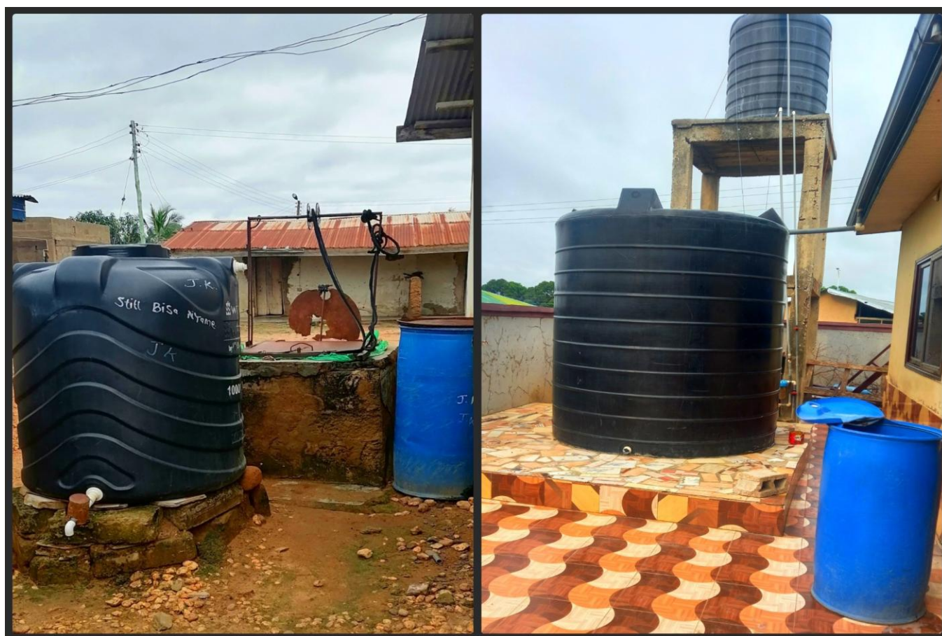
Figure 34: Samples of individual water supply with multiple storages in Bamboi
