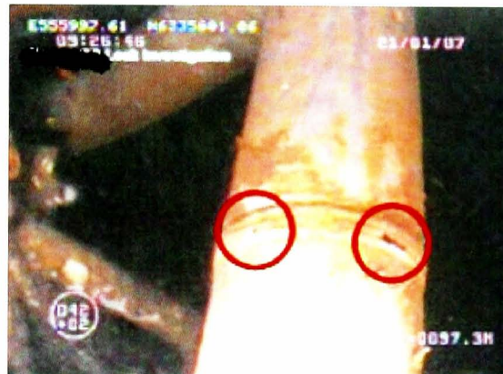
Figure 1-3: Leaking in subsea pipeline due to internal corrosion [16]
