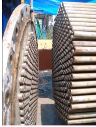
Fig. 5-27. Real-world heat exchanger cutting example showing the pipe segments separated from the partitioning baffle. Image from [212].
