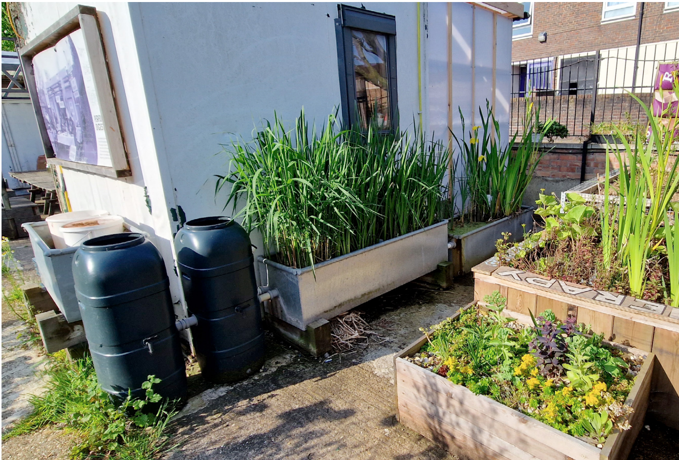
Figure 182 - The finished kitchen greywater system in 2023
