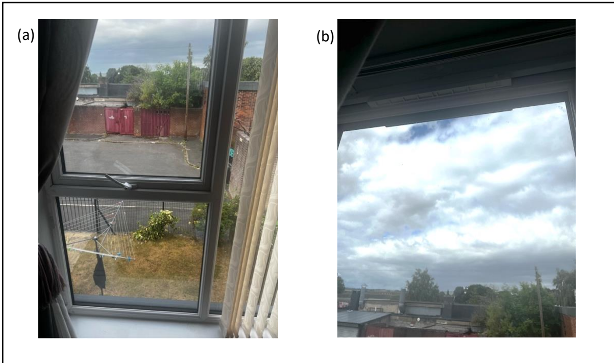
Figure 6.5 Ventilation controls in the social housing: (a) the double-glazing windows in one of the homes; (b) the trickle vents on top of the window in one of the homes
