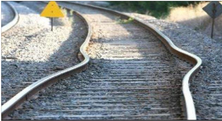
Figure 2.1: A typical track buckling failure. This failure mode can result from improperly managed longitudinal stress in a section of CWR . Image credit: Mandal-Lees [30]
