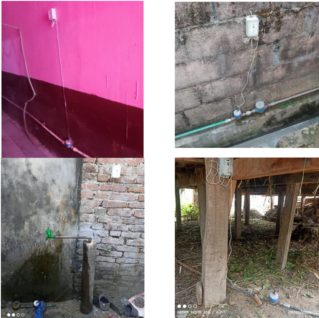
Figure 6.11: Example Household Smart Meter Installations
