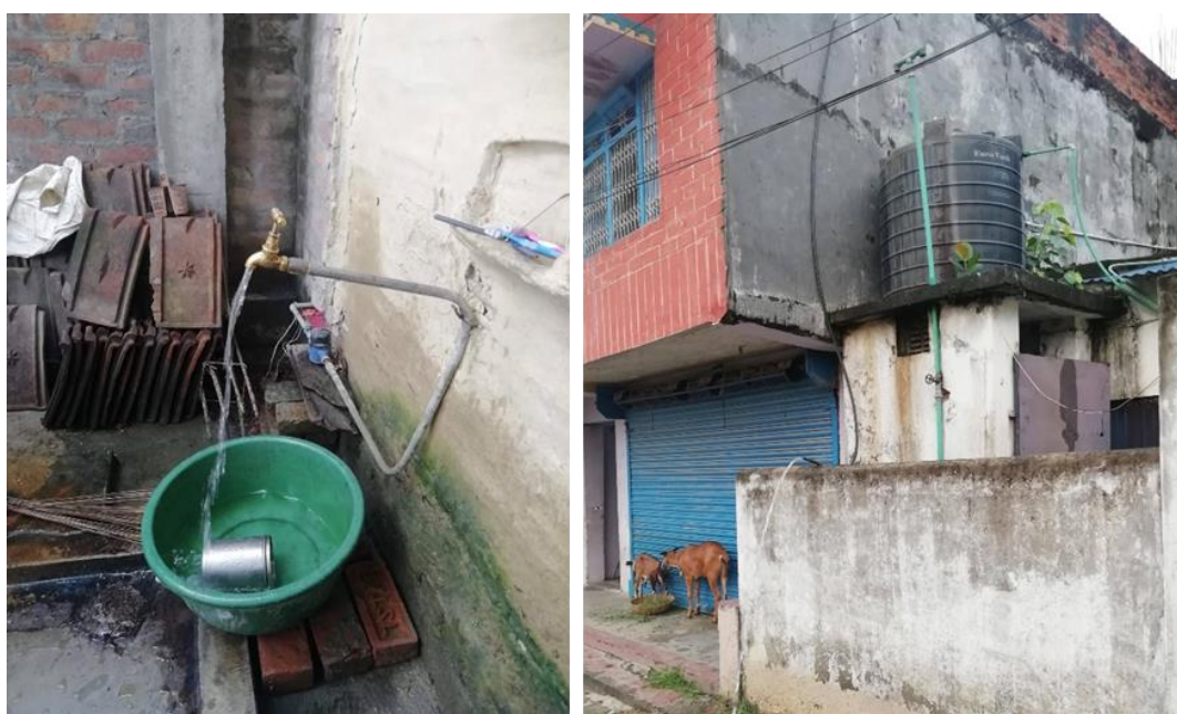
Figure 7.24: Typical Examples of a Yard Tap Arrangement vs a Fully Plumbed Installation
