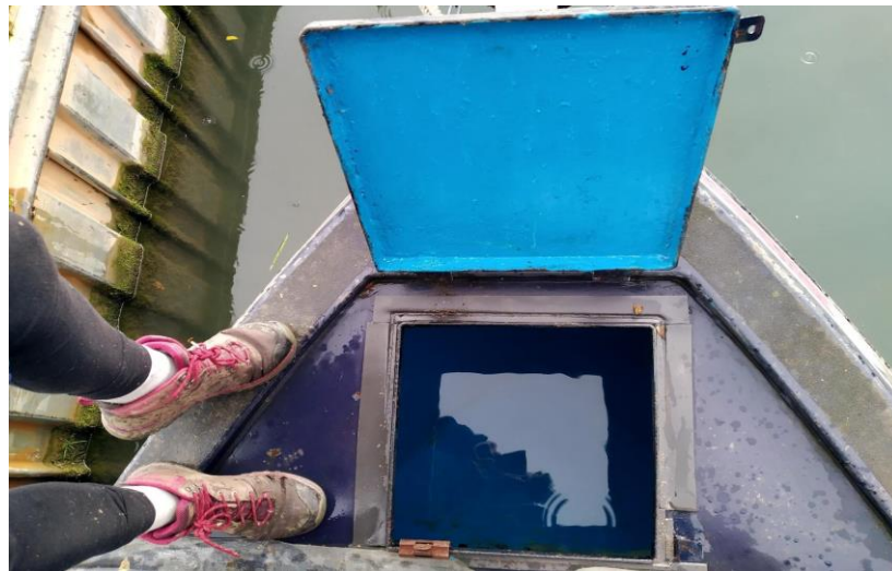
Figure 11: A2's integral steel water tank, painted with potable paint.
