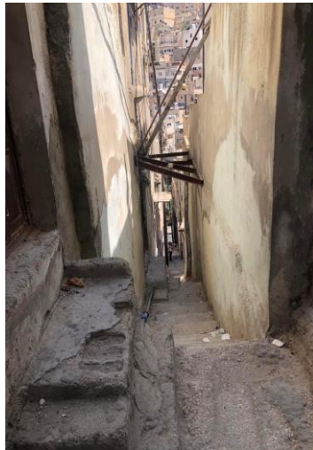
Figure 6.15: The parallel dangerous staircase next to staircase NO.7 site. Author ,2021
