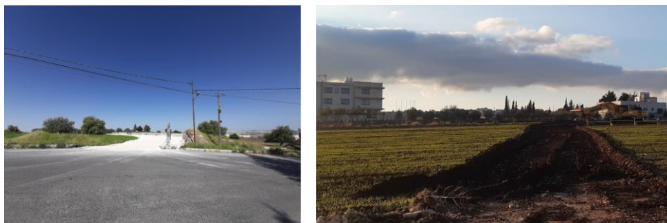
Figure 8.21: Destruction caused by GAM through the construction of a new road in one of the newly cultivated lands for the Al-Barakeh Wheat project. Source: Zikra for Popular Learning Organisation, 2021
