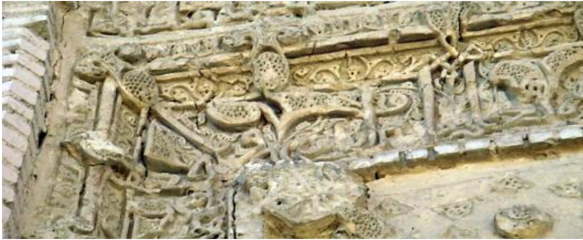
Figure 60: The relief and elaborate stucco decorations in Boomnama ornaments which have been executed in a stratified Do-Gacheh method, Gaar mosque, East of Isfahan, Seljuk period (Author).
