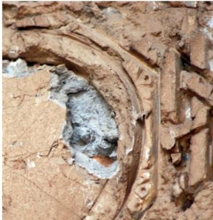
Figure 28: A close-up view of the plaster coat stucco with ash impurities and the base coat plaster on the part of the relief stucco decorations indicates that the plaster coat layer is applied to create the overall volume of the desired decoration. Then, with the application of one or several layers of the base coat plaster, the stucco operation is performed. mosque of Faruamad in Sabzevar, Ilkanid period (Author).
