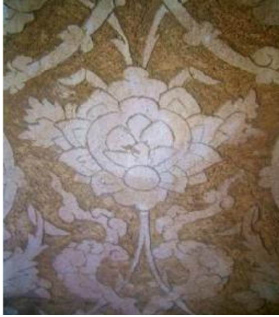
Figure 98: The grooves from the stage of scraping the design onto the 'white clay' preparatory layer adorn the unfinished Koshtebori decorations on the third floor of the Ali-Qapu palace, Safavid period, Isfahan, Iran (Author).
