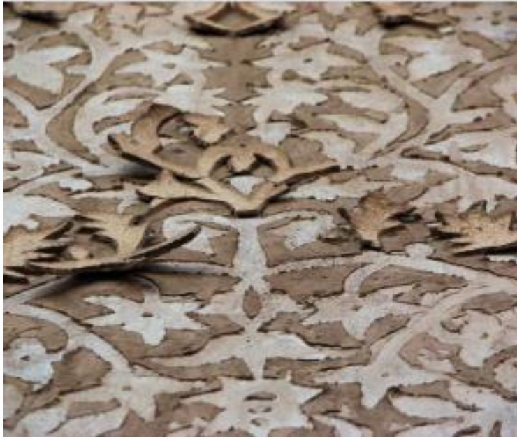
Figure 102: The separation and detachment of decorative stucco layers from the underlying surface substrate occur due to the differential behaviour of these layers towards moisture. This phenomenon is observed in the low-relief stucco decorations of the courtyard walls of a Gorji historical house, Yazd, dating back to the Qajar period (Author).
