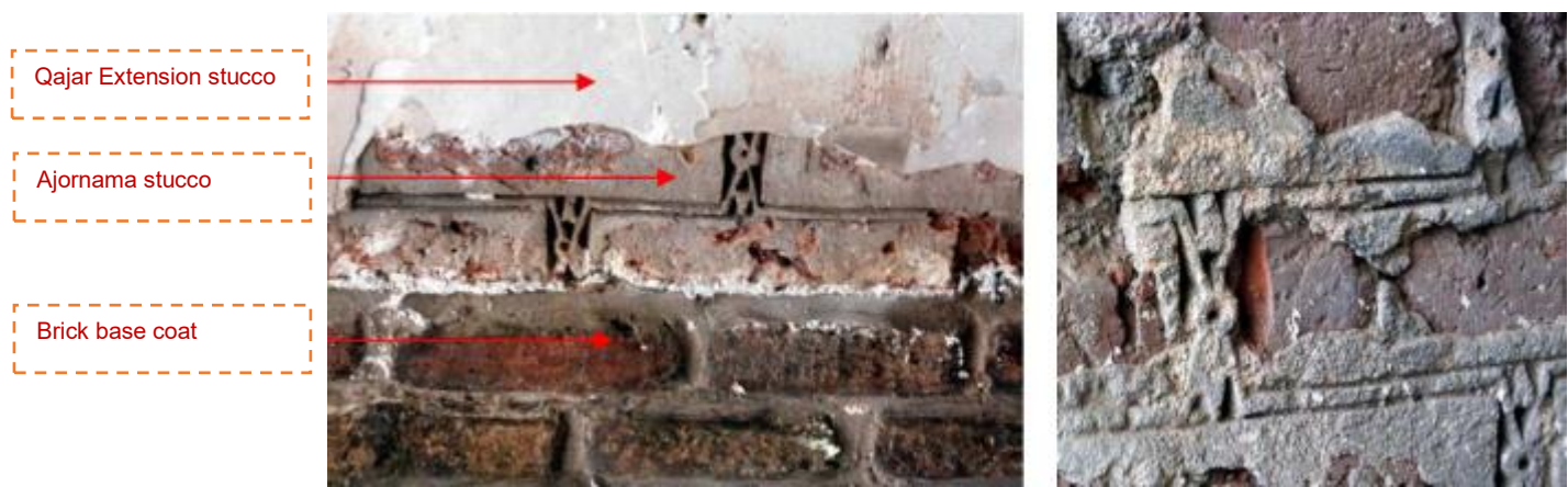
Figure 120: The Simulating patterned brick stucco, Zavareh Jameh mosque, decorations belonging to the Ilkanid period (Author).
