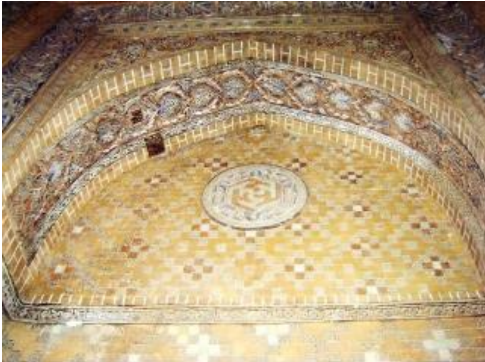
Figure 131: The variety of coloration in the stucco, Ajornama decorations, Sabz dome, Qom, Ilkanid period (Rahimi 2023).
