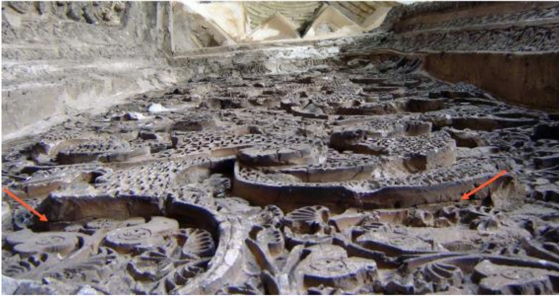
Figure 64: The close-up view of the relief stucco facade executed in the 'Double coat' method, featuring the separation of the surface stucco layer and the appearance of the boundary between the surface stucco background and the smooth base layer with underlying patterns, is evident with the red marks, Alavian dome, Hamedan (Author).
