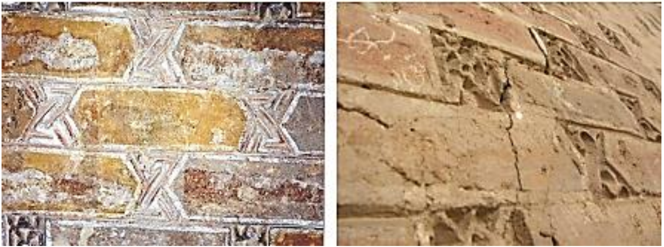
Figure 128: After the stucco carving stage in this method, further embellishment of the decorations was achieved through painting the surface layer of the stucco. In most cases, the colors used include two dominant hues: Mustard yellow to simulate bricks and white for areas intended to represent gypsum facades. Traces of remaining paint on two samples of Ajornama decorations, Sultanieh dome, Zanjan, Ilkanid period (Author).
