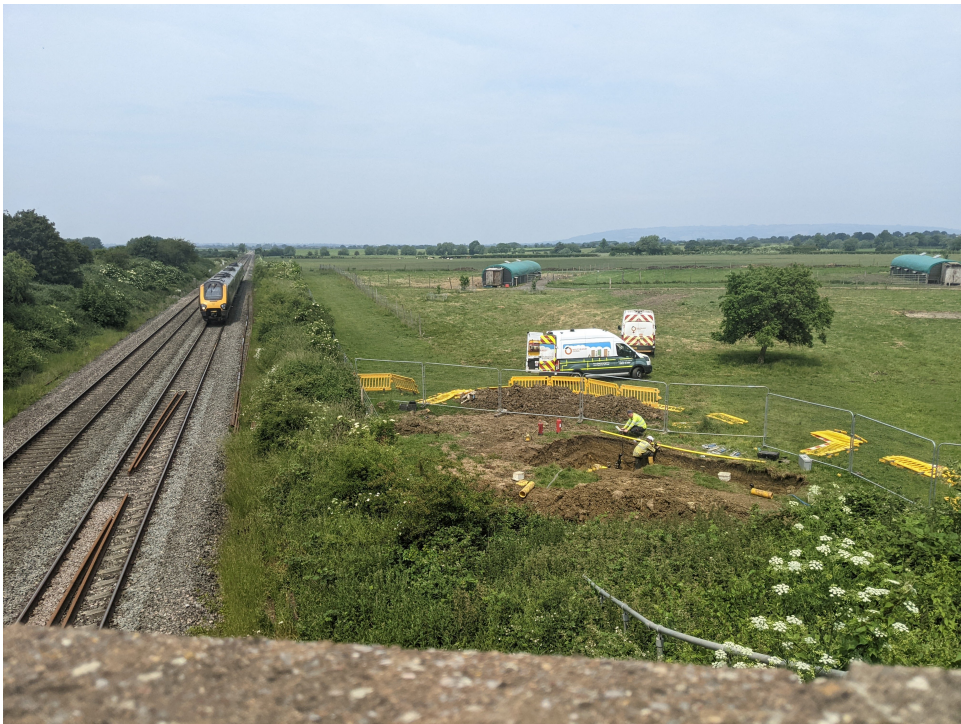
Figure B.1: Image of gas leak site works taken on 12th June 2023.
