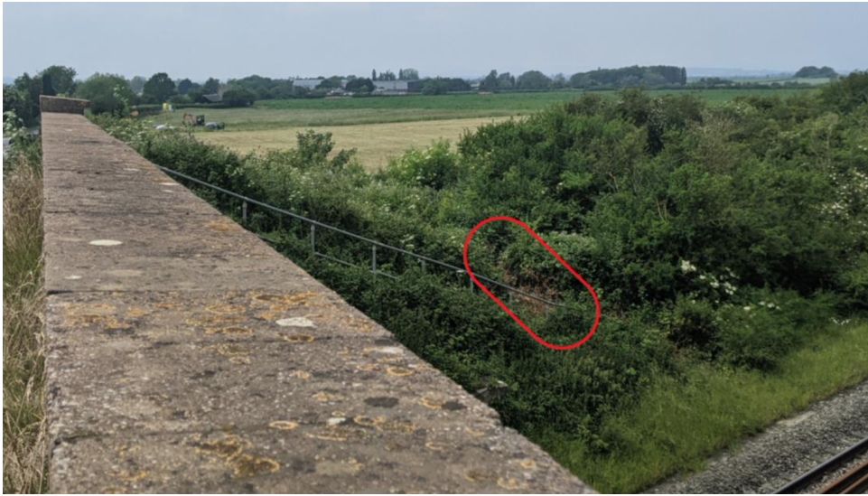
Figure B.2: Image of dead vegetation (circled in red) at gas leak site taken on 12th June 2023.
