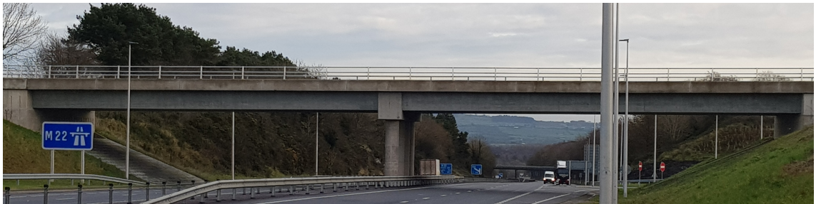
Figure 5.2: A two-span beam-and-slab bridge example from Northern Ireland. The same bridge that is showcased in Chapter 3.
