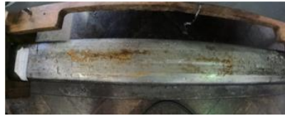
Figure 6. 15: Example of railhead images for rust day2 + water. Horizontal with camera-railhead distance \approx 450\text{mm} distance (L) and vertical with camera-railhead distance \approx 700\text{mm} (R) (21-04-22)
