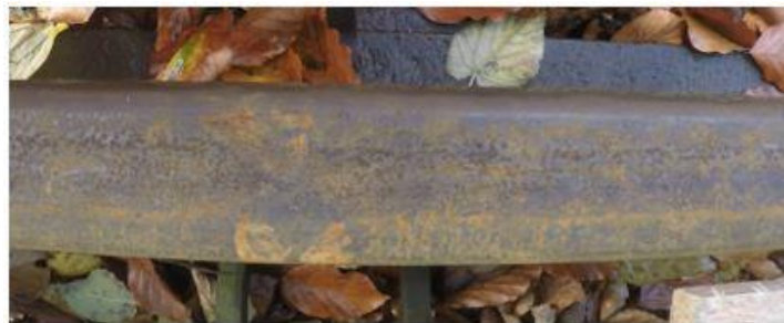
Figure 6. 38: Example of oxidised railhead image captured infield
