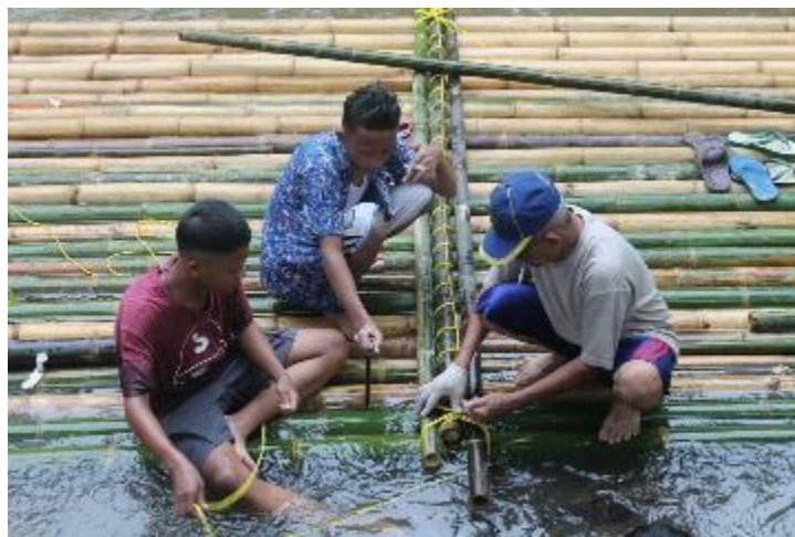
Figure 172 The making of bamboo raft over the river buoyancy, by Indrawan Prabaharyaka, 2017.
