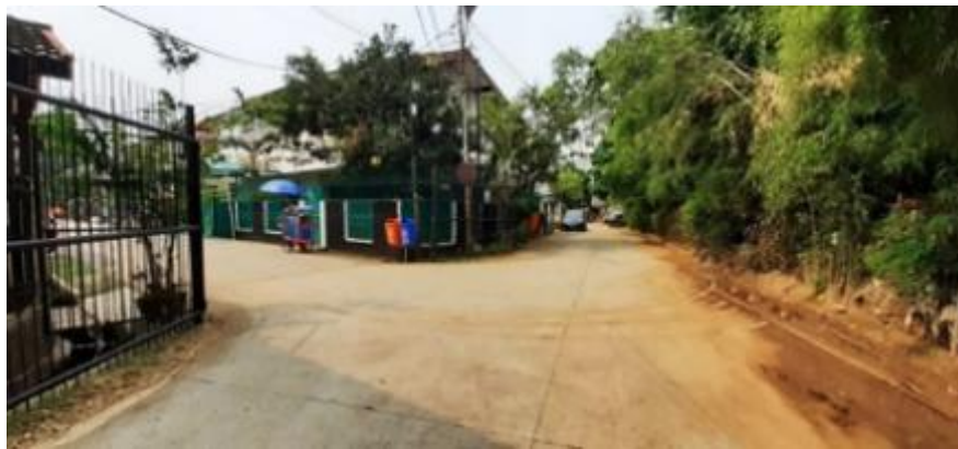
Figure 203 Cemented concrete road covered the ruined asphalt surface due to exposure to wetness in the rising surface of river water next to the street, by author, 2021/08/19.
