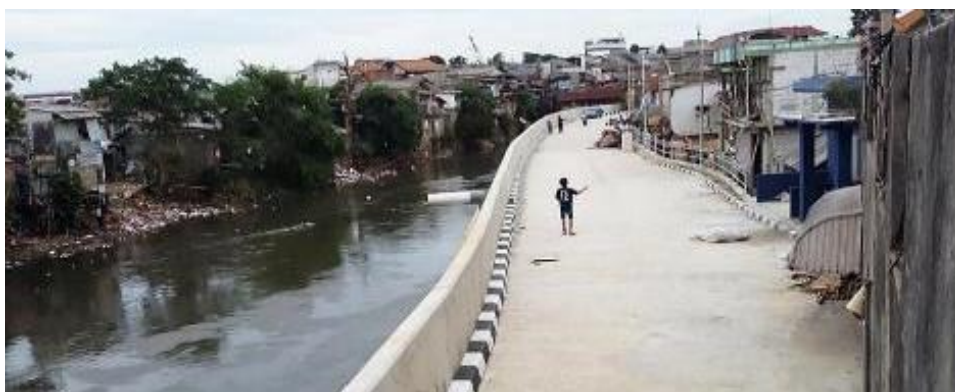
Figure 197 Newly built floodwall and road embankment on the side of Garuda residential cluster, another side of the riverbank of Tanah Rendah, by author, on 2018/10/06.
