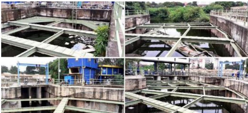
Figure 182 Abandoned underground tunnel designed to connect water flow of Kali Ciliwung with the East Flood Canal that relied on the land acquisition process, by author, 2021/03/16.
