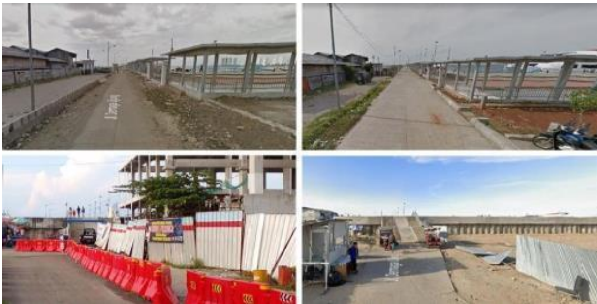
Figure 141 The emerging seawall from Google View in April 2013 and 2015 (top), with April 2019 (bottom), compiled by author, in 2021.
