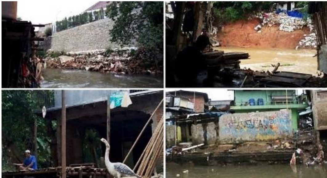
Figure 198 Continuous ruining and rebuilding of the eroding riverbanks affecting the low-lying settlement, by author, 2017/11/26.
