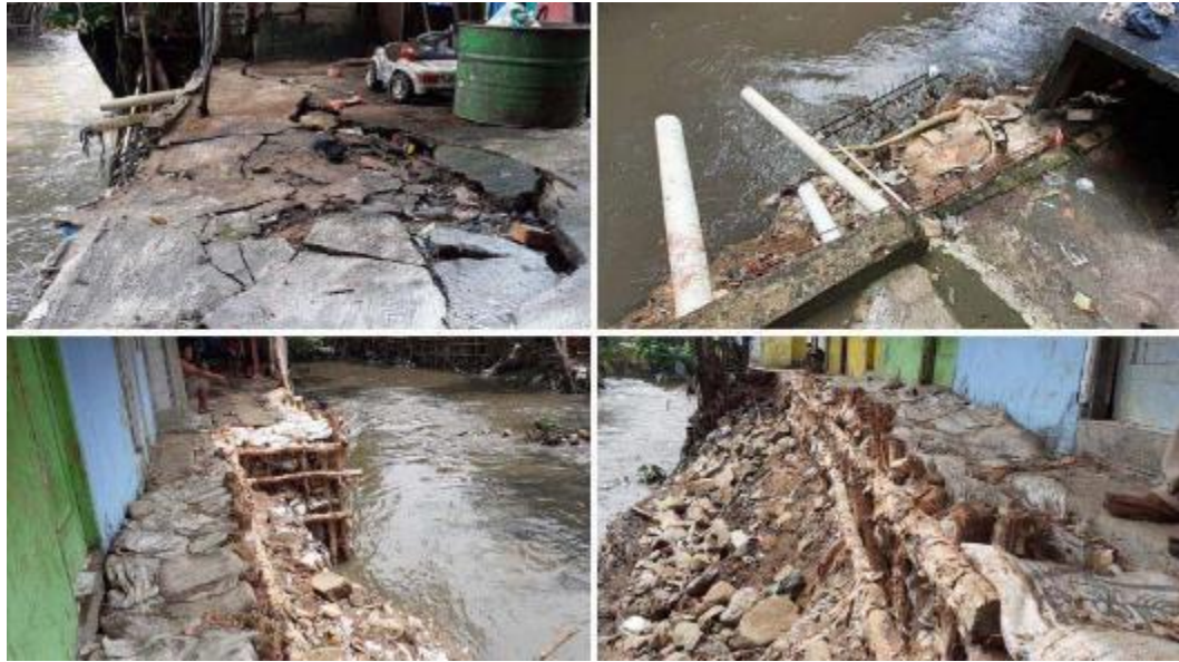
Figure 188 Makeshift structure to retain cracking edge and eroded part of riverbank, by author, 2021/03/02.
