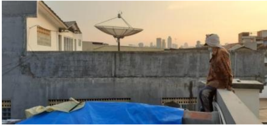
Figure 174 Kumis took a rest on a gable end after a day of repairing a leaking rooftop of one of the houses in settlements near the Kali Ciliwung, by author, 2021/07/02.
