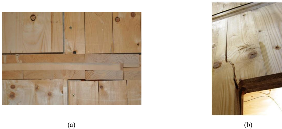
Figure 2.9. Timber panels damage observed in the quasi-static test of CLT buildings: (a) embedment of wall panels into floor panels (b) cracking in the corner of large opening [2.22]
