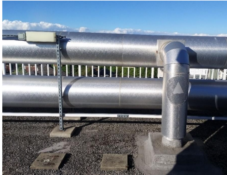
Figure 3-2: Insulated piping system at the University of Leeds
