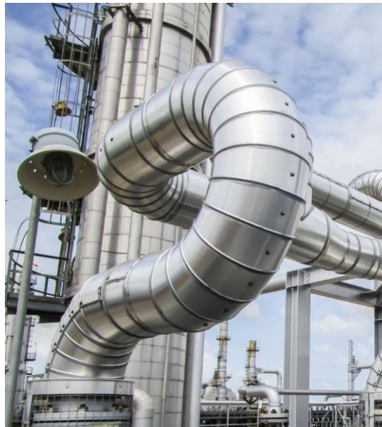
Figure 3-1: Thermally insulated pipe and vessel in an oil refinery [64]
