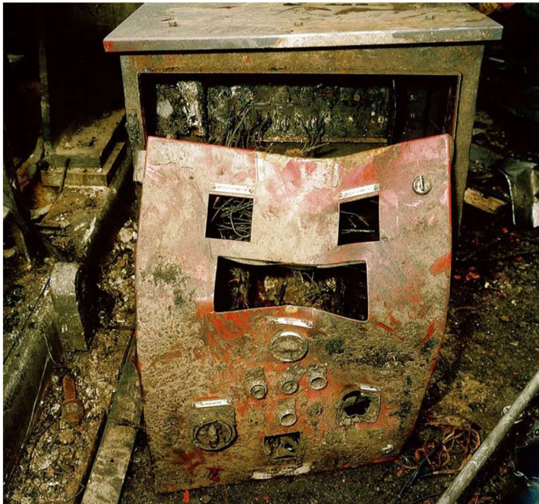
Figure 13 - Buncefield diesel pump electrical control box [84]
