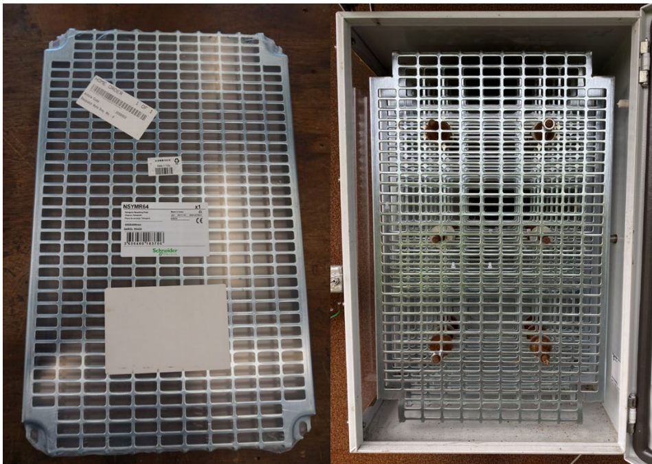
Figure 32 - Chassis plates used for congestion, as received and fitted into the wall box
