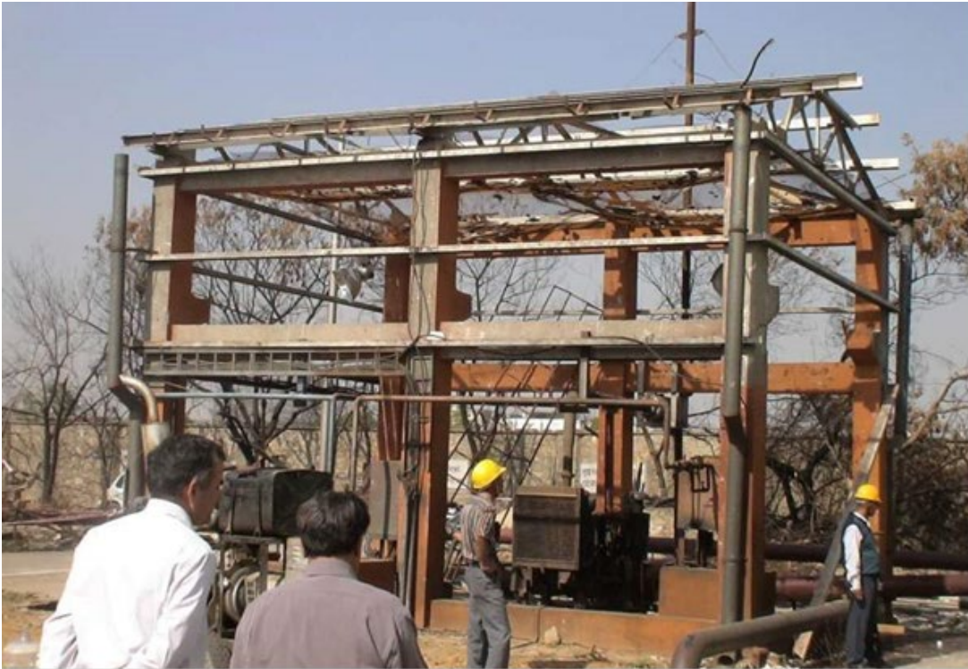
Figure 2 - Remains of the pump house at Jaipur [12]
