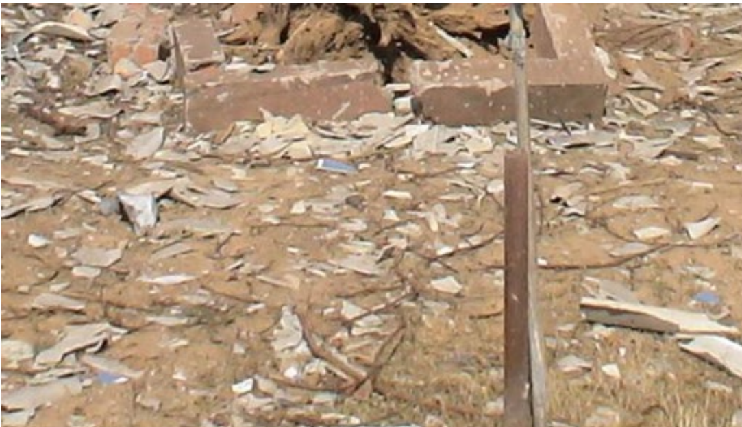
Figure 3 - Fragments of cement cladding panels around the pump house at Jaipur [12]
