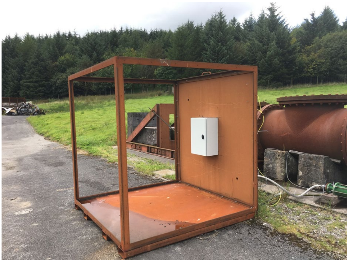
Figure 30 - Steel frame rig with electrical control box mounted
