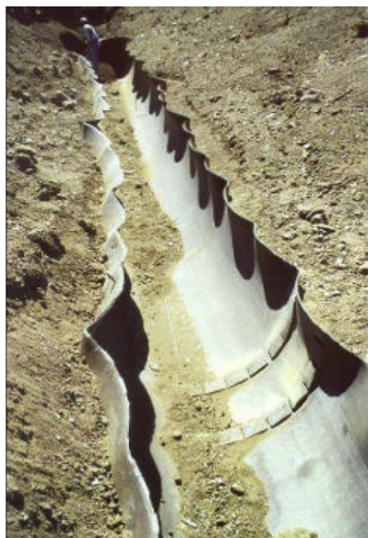
Figure 2-1 Ruptured pipeline. Reproduced from (28)
