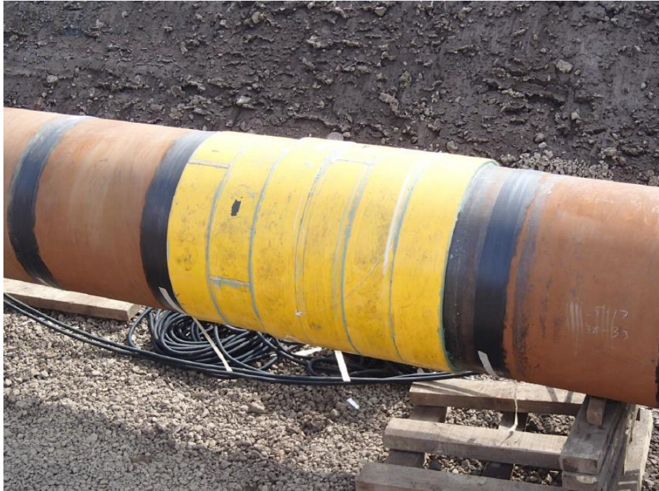
Figure 3-5 Photograph showing a crack arrestor installed on the reservoir section
