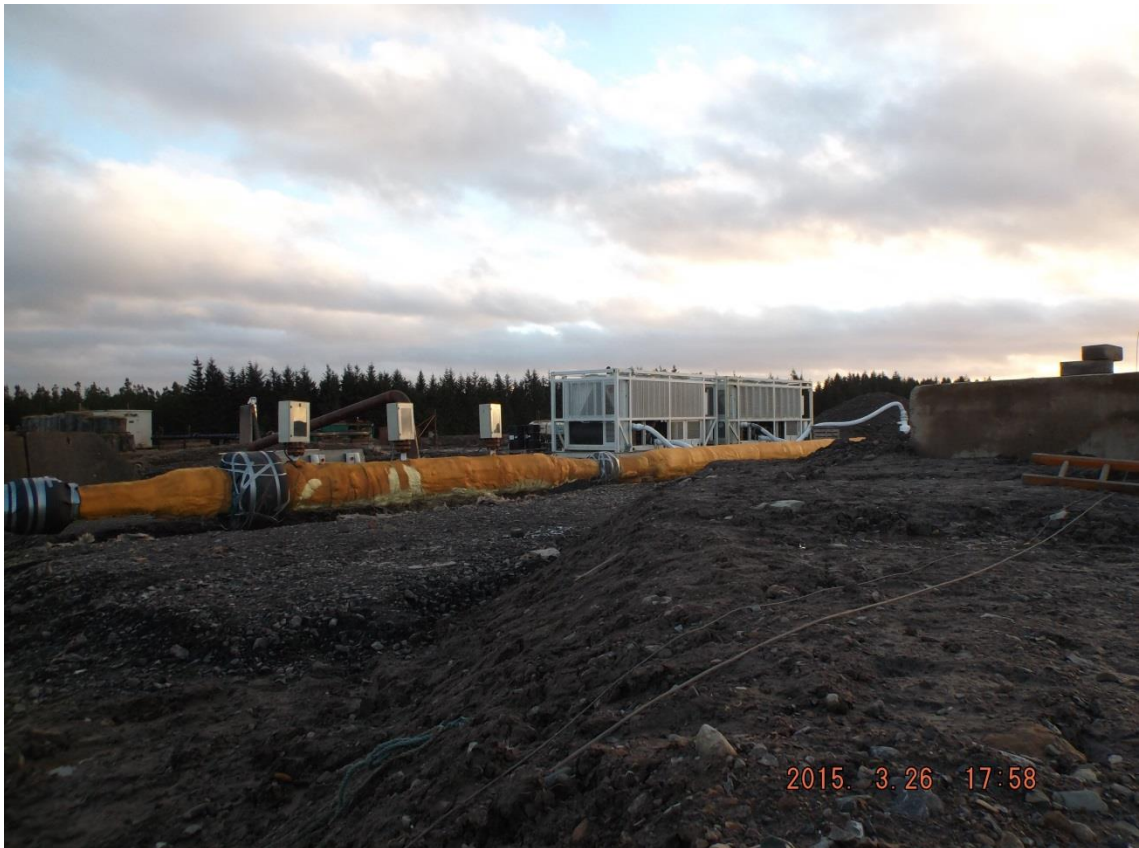
Figure 3-10 Test loop with chillers installed prior to test
