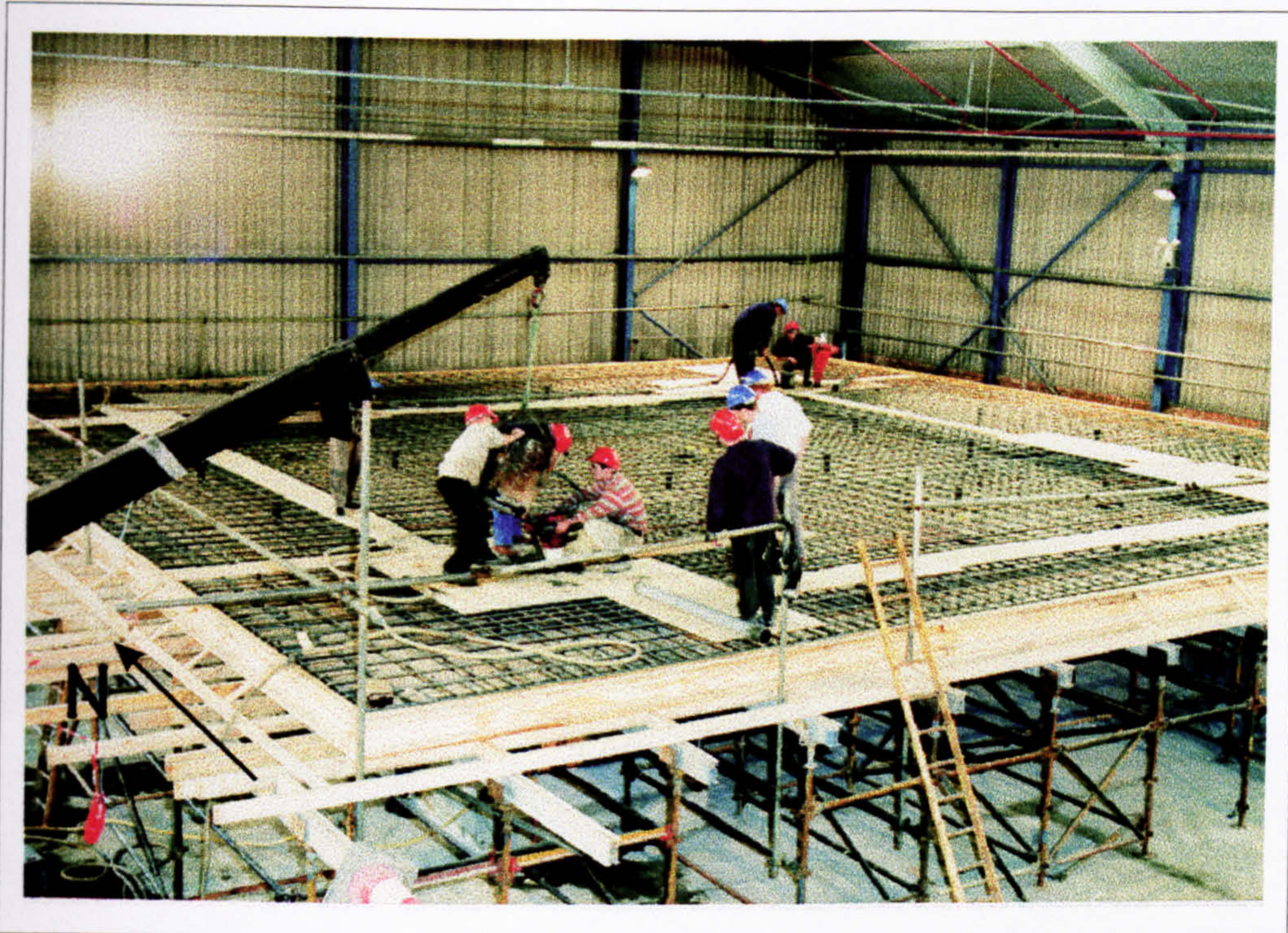
Figure 5.39: Structure B - Reinforcement placement and casting of columns prior to slab concreting (courtesy of Taywood Engineering Ltd).
