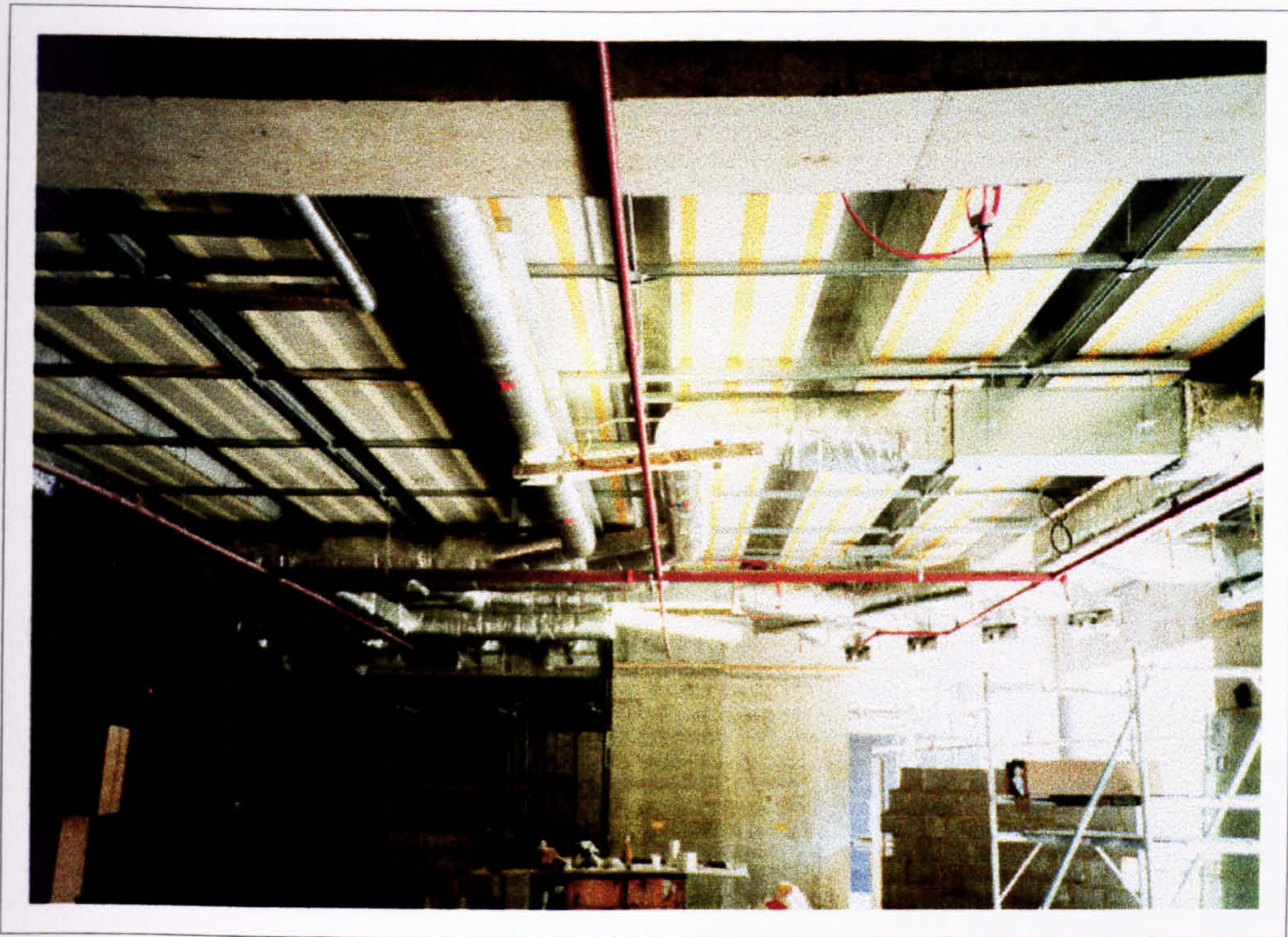
Figure 5.78: Structure C (Clad) - Installations and piping underneath the floor.
