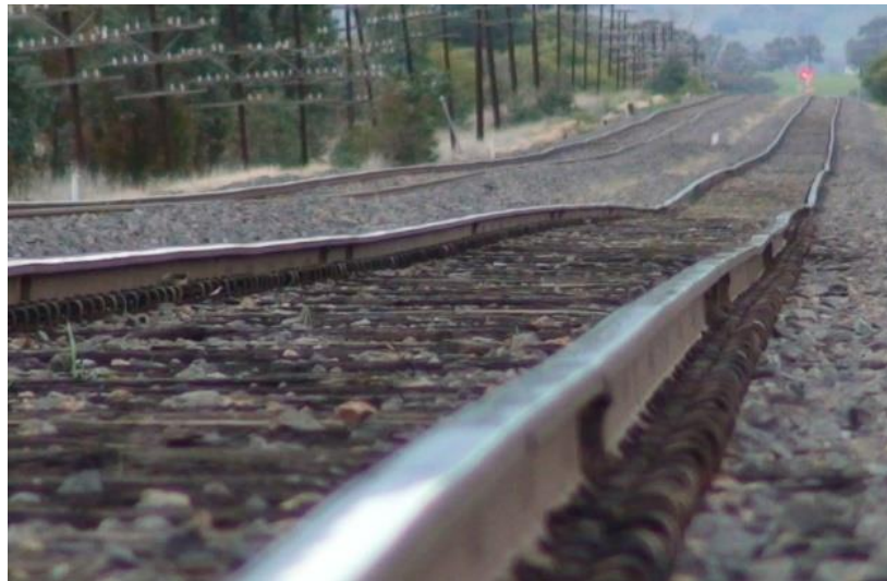
Figure 2.3 Visible geometric defects in a railway track: alignment (above) and longitudinal levelling (below)
