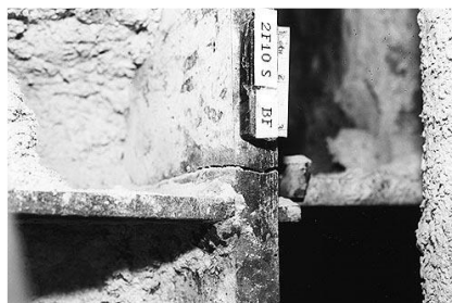
c) Fractures through column flange.
