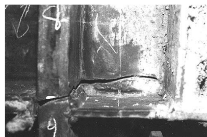
d) Fracture progresses into column web.
