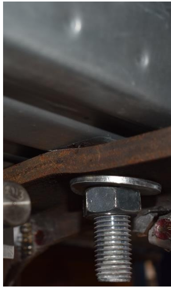
c) Bolted studs' failure.
