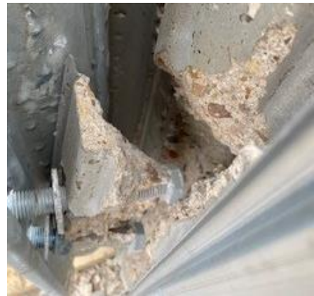
b) Concrete cone failure.
