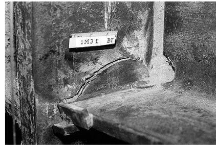
b) Column flange fracture.
