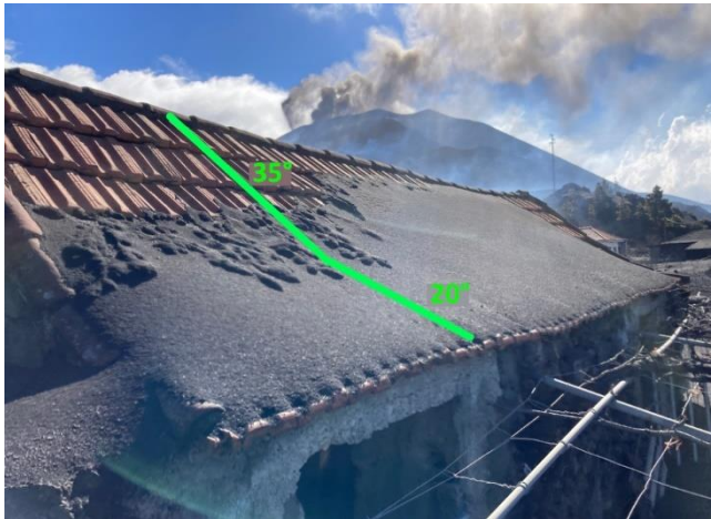
Fig. 3-11 Tephra deposit on a roof in Tacande, La Palma, December 2021 during the Cumbre Vieja eruption. Tephra has slid on the steeper part of the roof ( \sim 35^\circ pitch) but accumulated on the lower, shallower part ( \sim 20^\circ )
