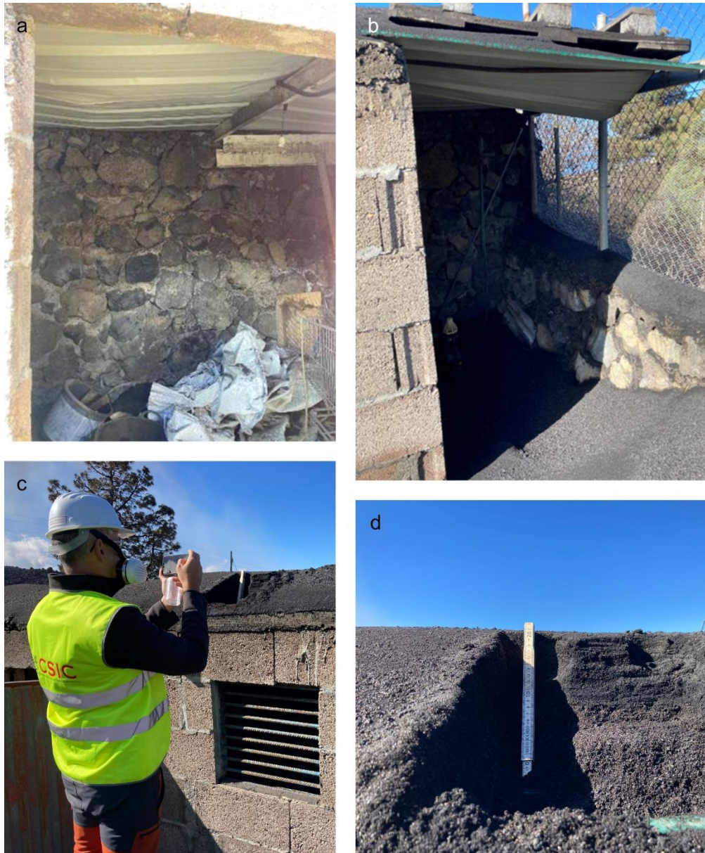
Fig. E-7: Outbuilding T10 in Tacande (location shown in Fig. E-4) showing a) and b) Buckled metal sheet roofing, c) and d) Tephra deposit on the roof
