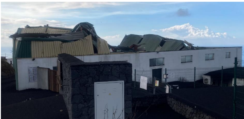
Fig. 6-2 Partial roof collapse at the wrestling arena in Las Manchas
