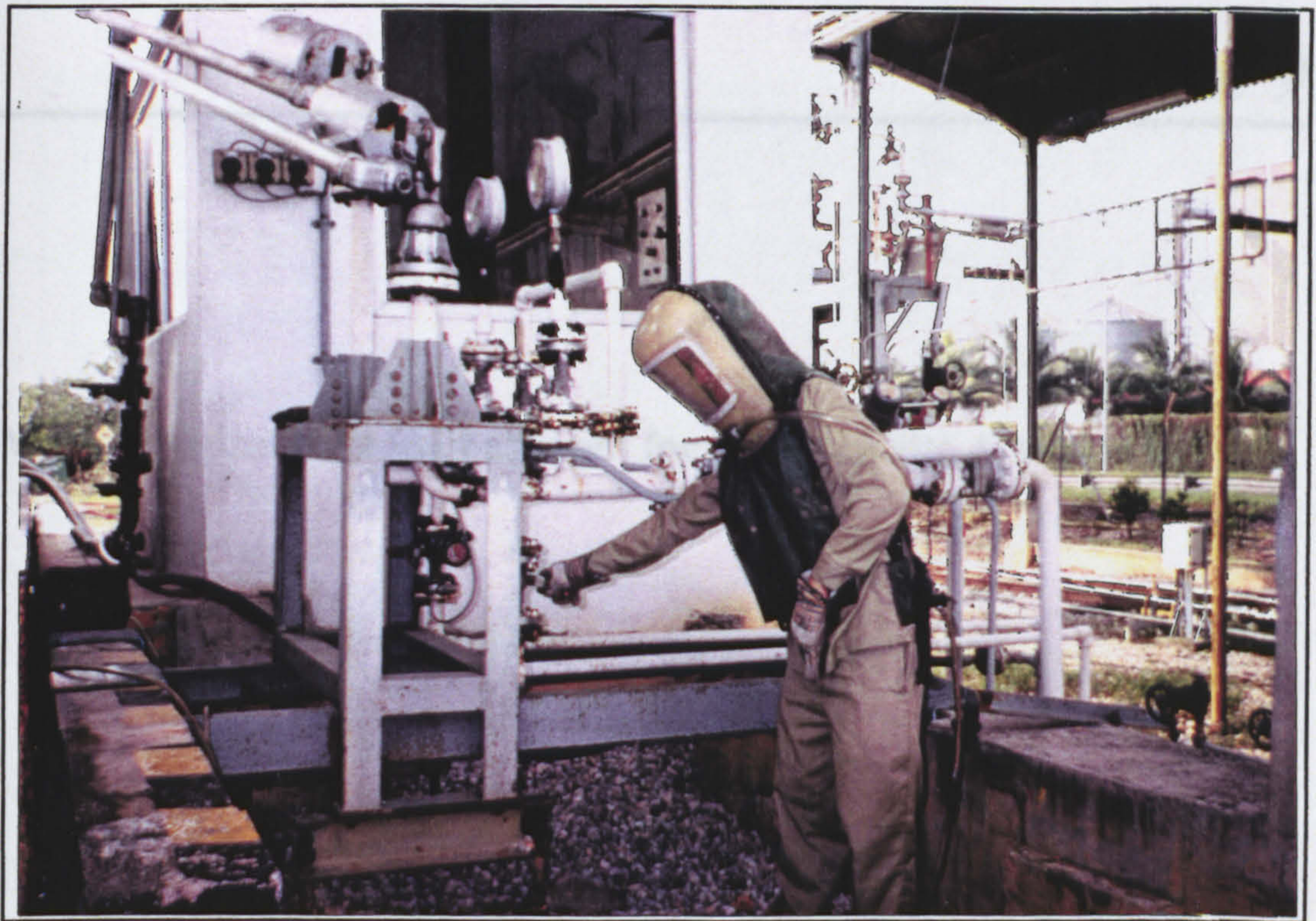
Figure A8.7. Chiksan arm s and flexible hoses connection at Site B
