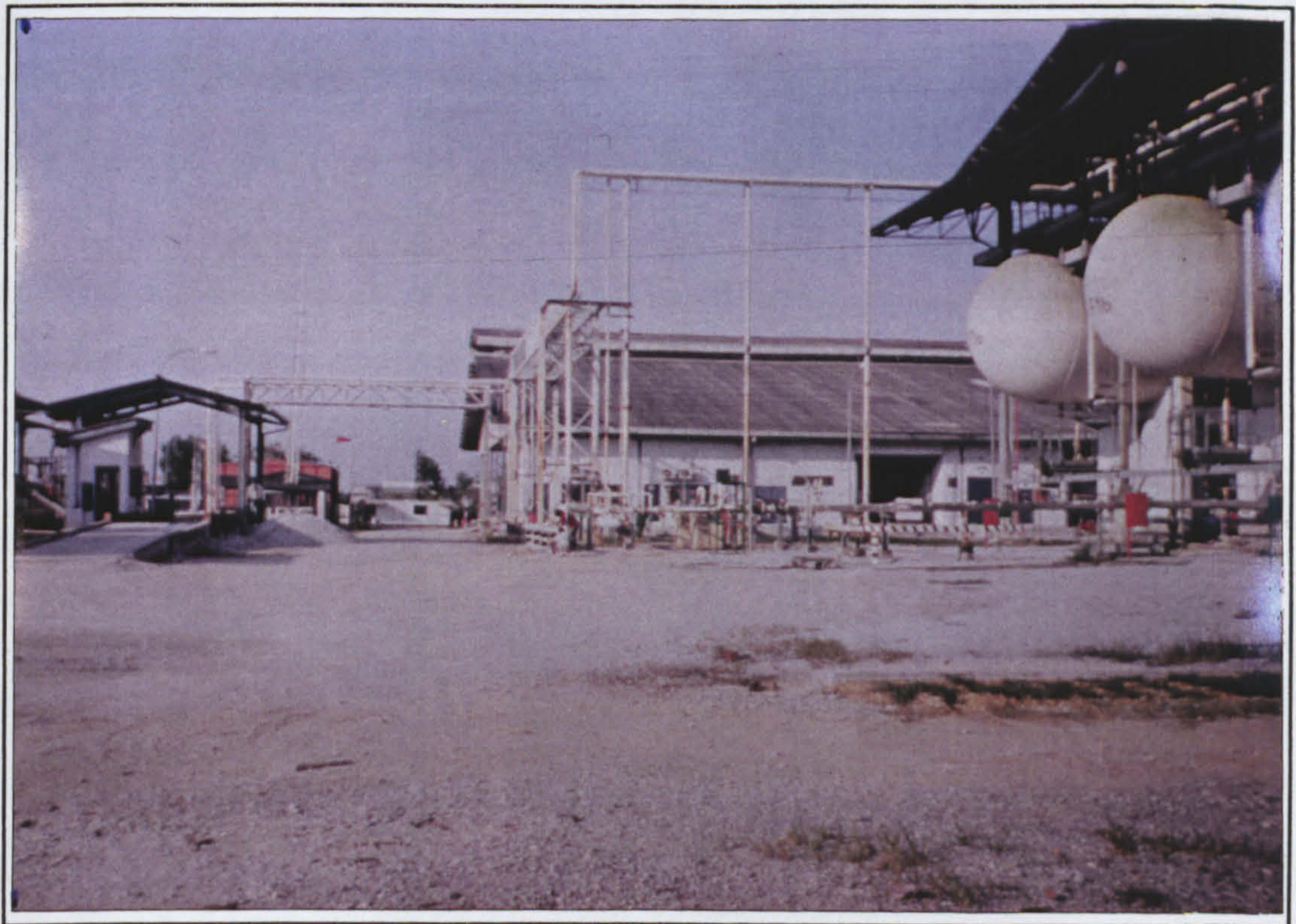
Figure A8.8. Piping arrangement from road tanker loading bay to ammonia bulk tanks at Site B
