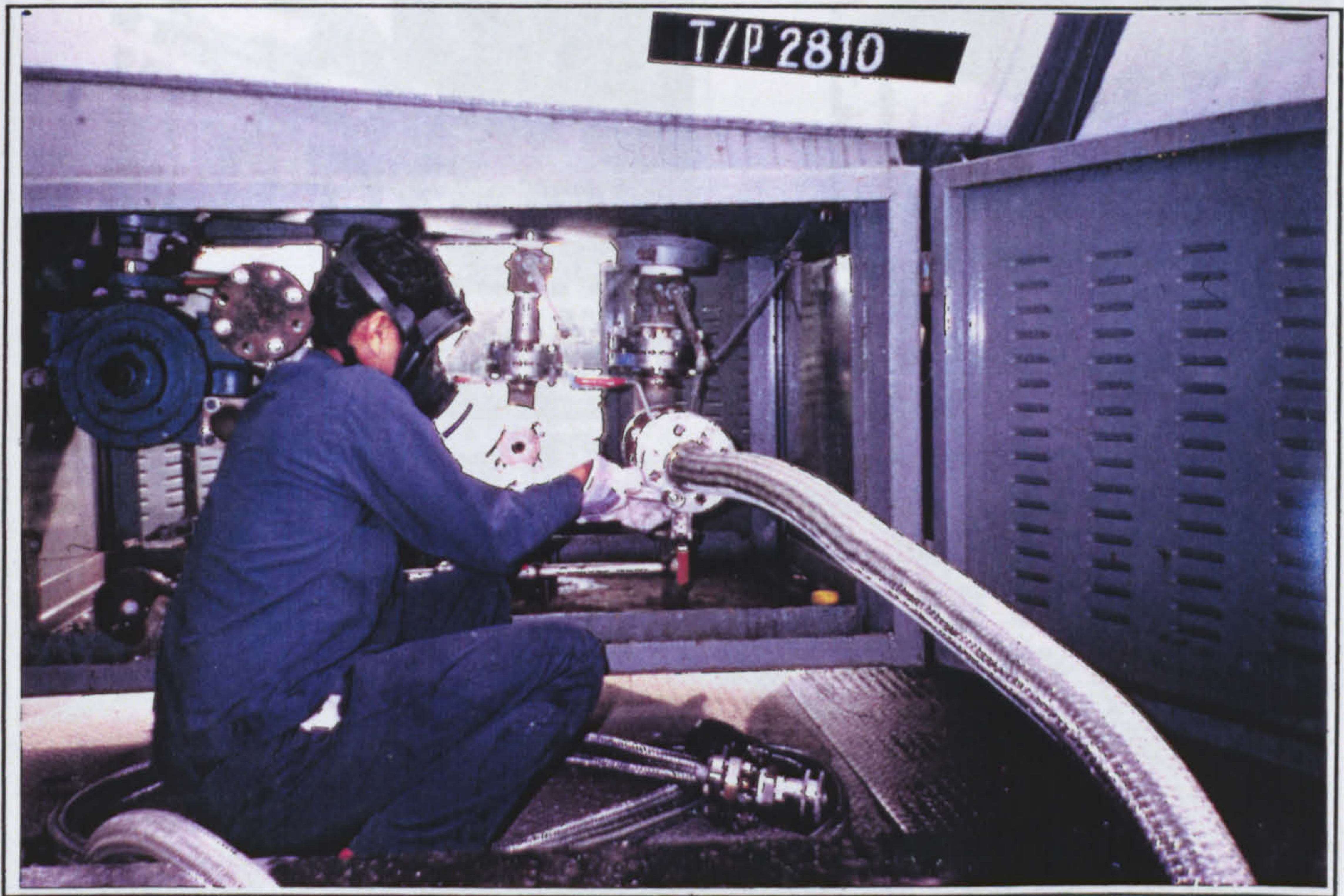
Figure A8.5. Maintenance fitter connecting flexible hoses for ammonia road tanker loading at Site B
