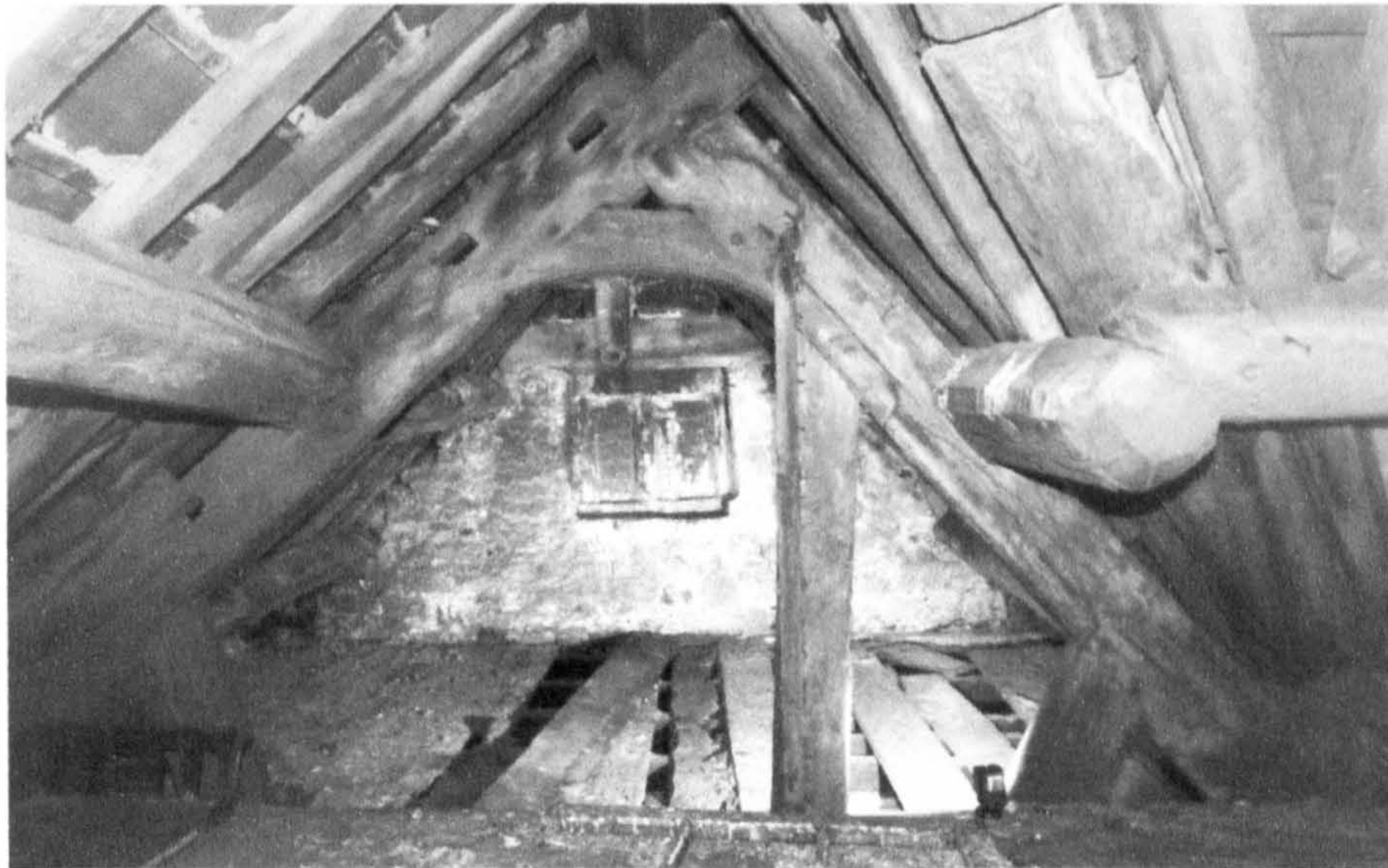
Fig. 4 The Red Lion (former Hall House): the roof of the eastern pile in 1999.
