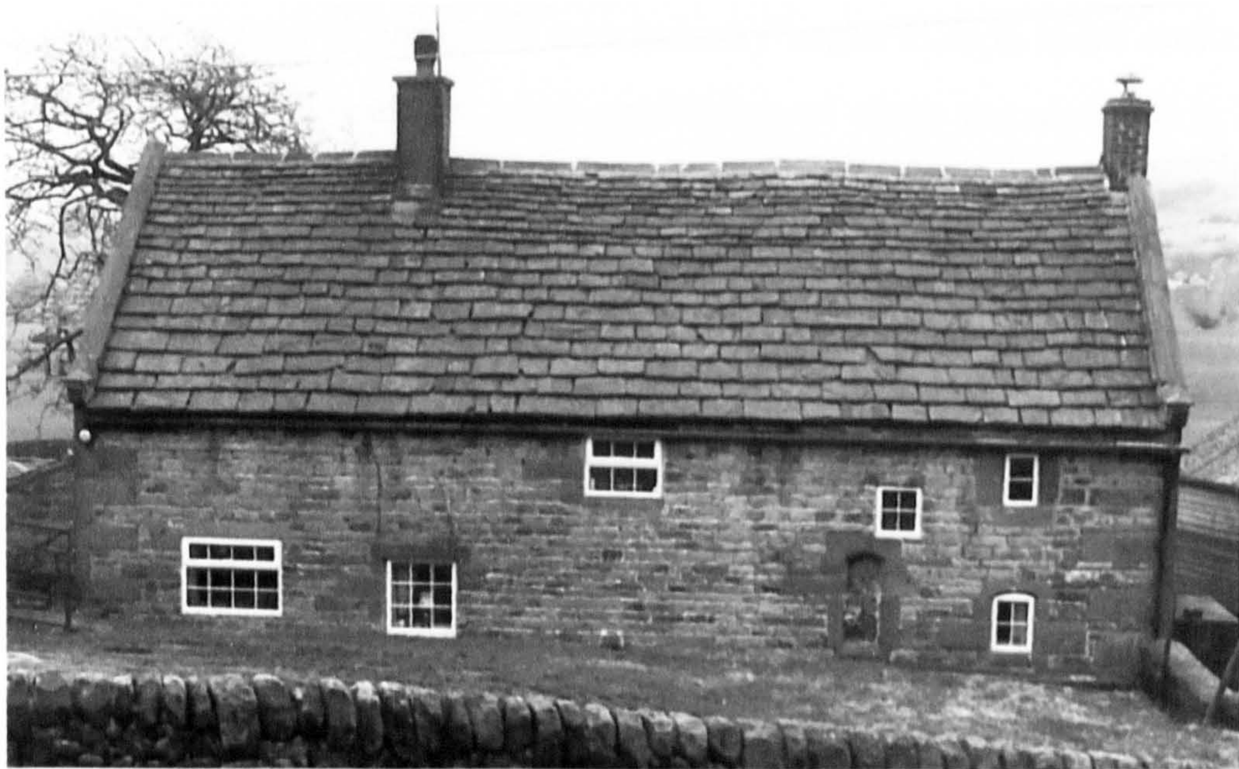
Fig. 5.5 Buxton Brow: stone tiling on the rear of an early-eighteenth century house
