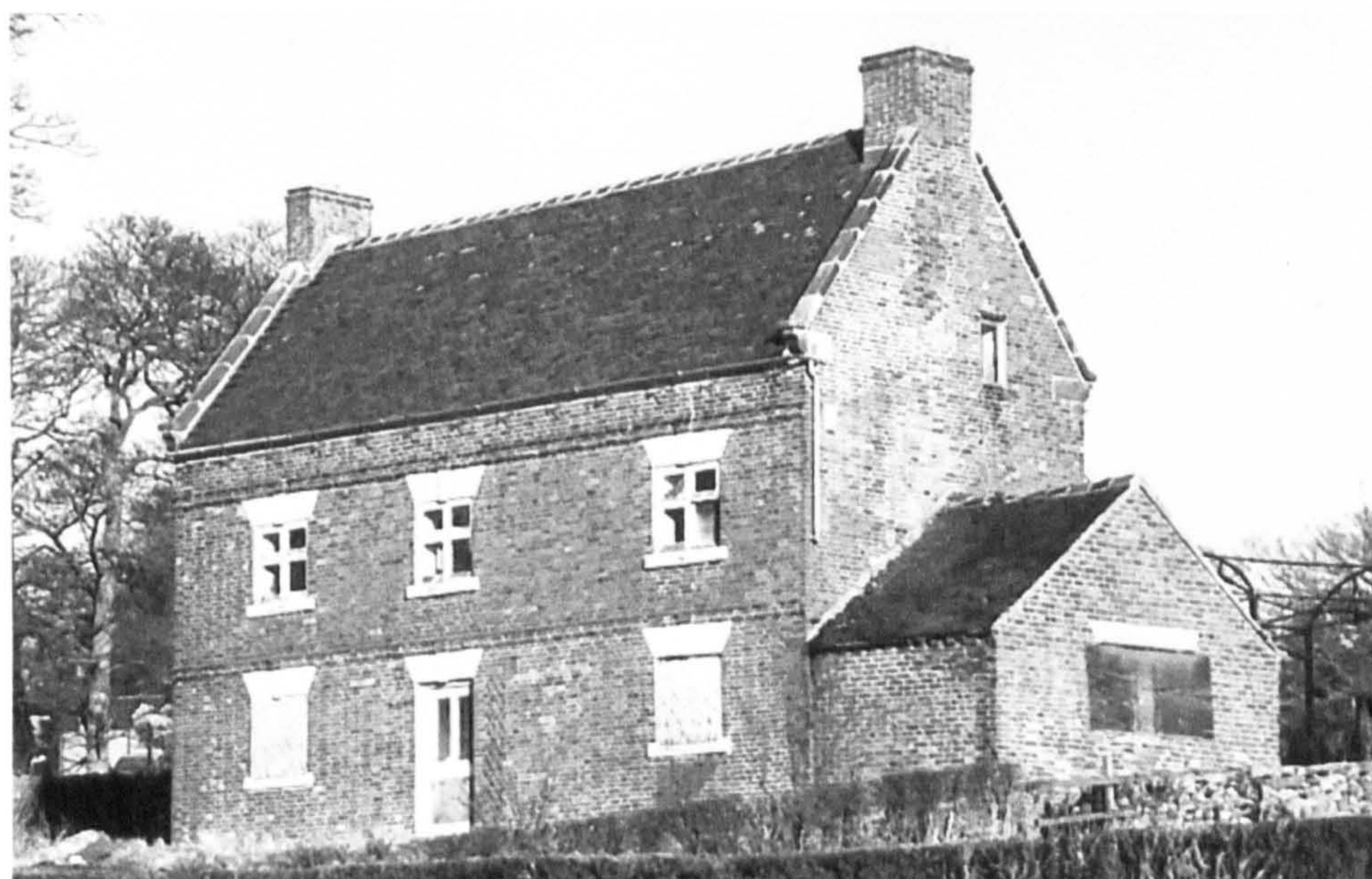
Fig. 6.83 Trees, Longsdon: (above) from the southeast before restoration in the 1990s. The original door position is visible to the right of the present front door. (below) the ground plan.
