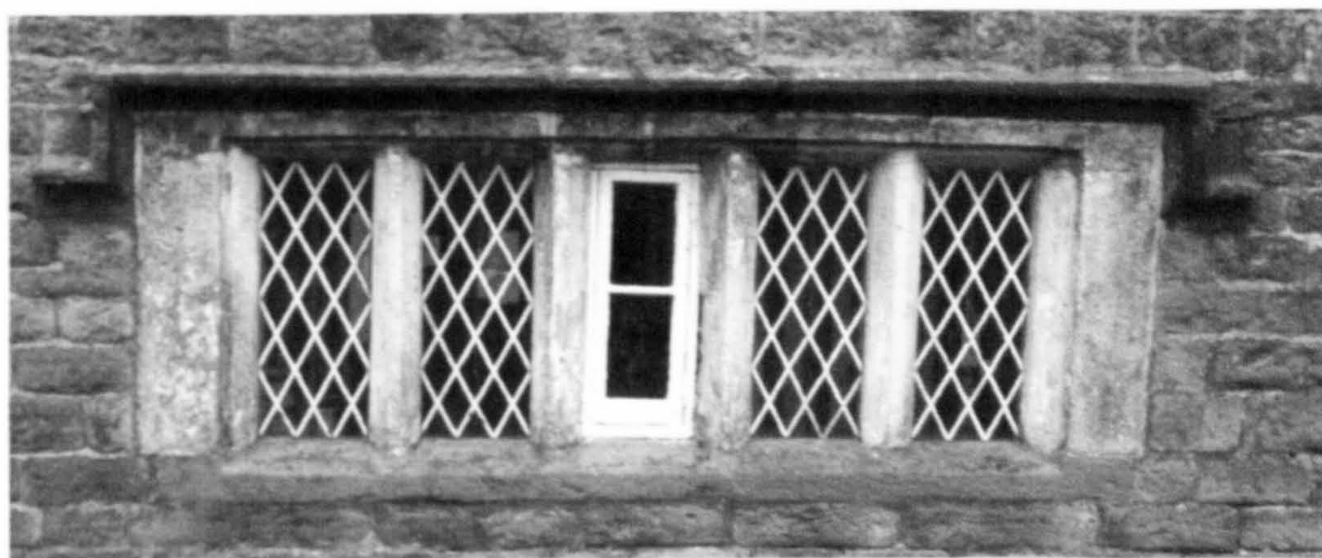
Fig. 6.146 Goldsitch, Heathylee: diamond paned glazing with its original glazing bars. The lead has recently been painted white
