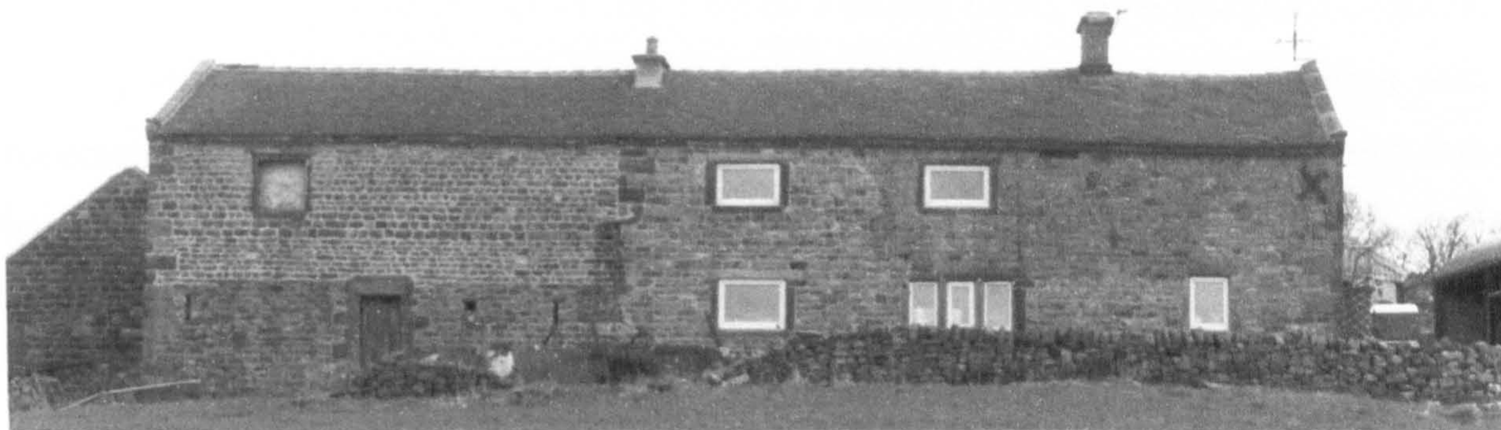
Fig. 6.76 Shaw, Heaton: (above) from the west with its nineteenth century barn; (below) Shaw: the ground plan of the seventeenth century house.
