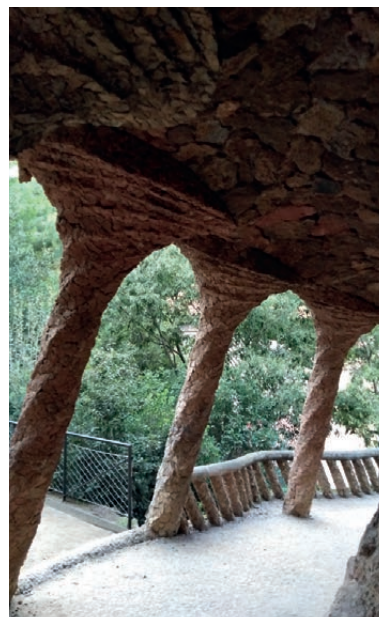
c) Tilted columns
