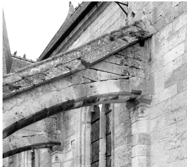
Figure 3.9: Failure due to slippage in a form-resistant structure: sliding near the head of a flying buttress at Saint-Julien in Royaucourt (after [47]).
