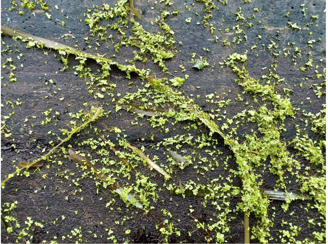
Figure 18. Lee navigation, Tottenham. Aquatic plant life sticks to the interior of a lock chamber wall as the lock is emptied and the water drops. 2022.
