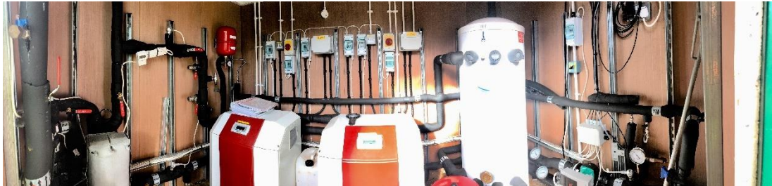
Figure 150 - GSHP Equipment in Outdoor Container (Boon et al. , 2019)
