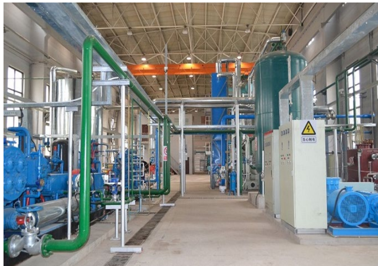
Figure 2-7 Hebei Langfang 1.5 MW SC-CAES pilot plant (Wang et al., 2017)
