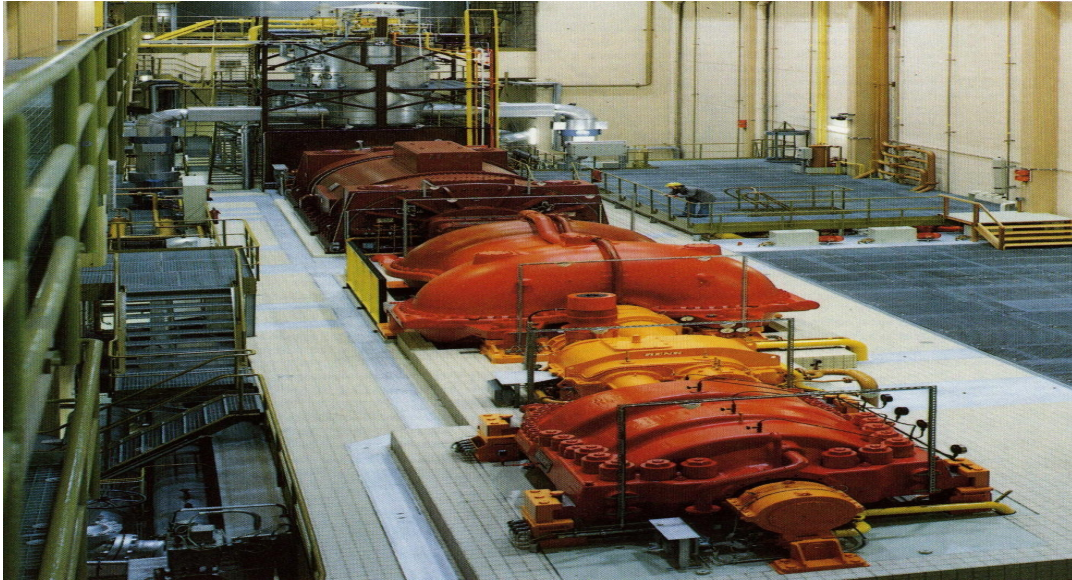
Figure 2-1 Huntorf CAES plant (Budt et al., 2016)
