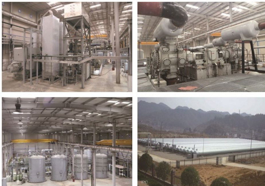
Figure 2-6 Guizhou Bijie 10 MW AA-CAES pilot plant (Wang et al., 2017)
