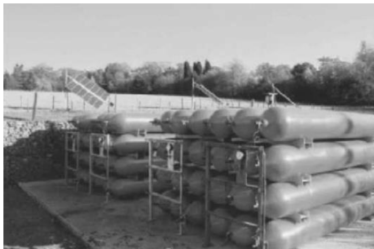
Figure 2.3. Tanks of compressed hydrogen at the HARI project, West Beacon farm, Loughborough. 2856 Nm 3 of hydrogen is stored at 137 bar, providing the farm with around three weeks of storage (3.8 MWh). Image: [27]. Reproduced by permission.
