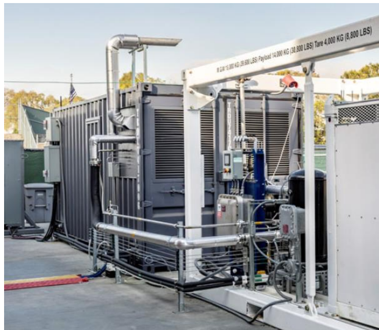
Figure 2.7. rSOC energy storage system demonstrated at Boeing Huntington Beach. [24]. Reproduced by permission.
