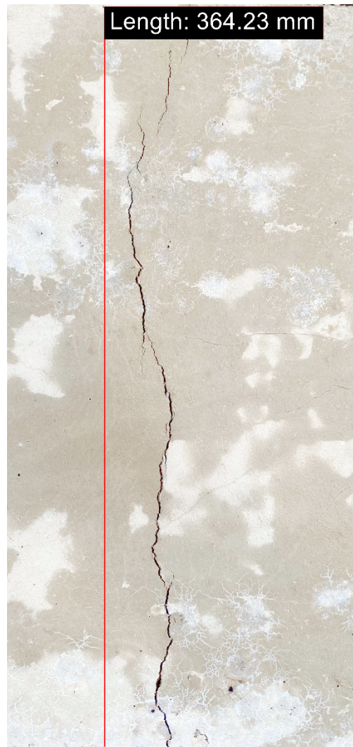
Figure B.2: IC crack length at 24 hours of plain concrete.
