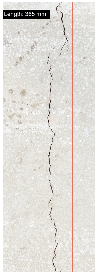
Figure C.31: IC crack length at 24 hours of plain concrete.
