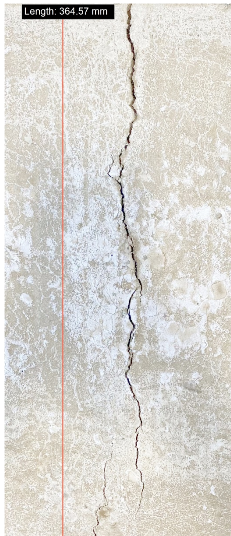
Figure D.22: IC crack length at 24 hours of plain concrete.
