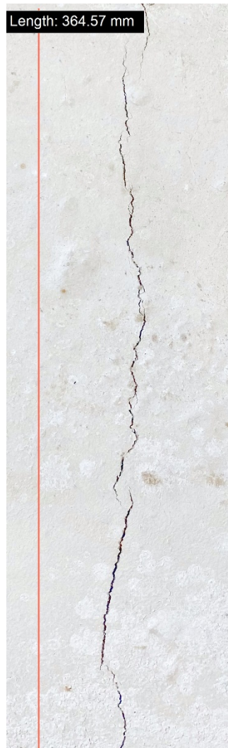
Figure D.7: IC crack length at 24 hours of plain concrete.
