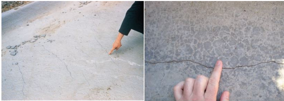
Figure 2.1: Typical plastic shrinkage cracks [5].
