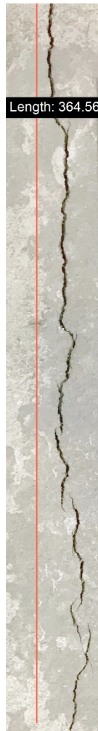
Figure C.19: IC crack length at 24 hours of plain concrete.
