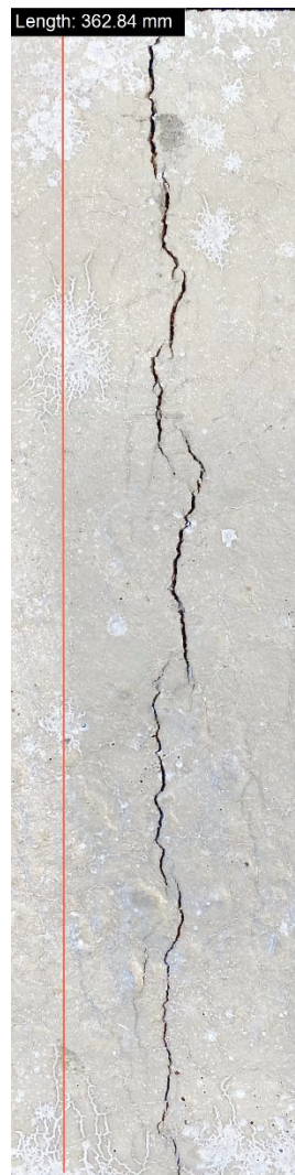
Figure D.37: IC crack length at 24 hours of PC.
