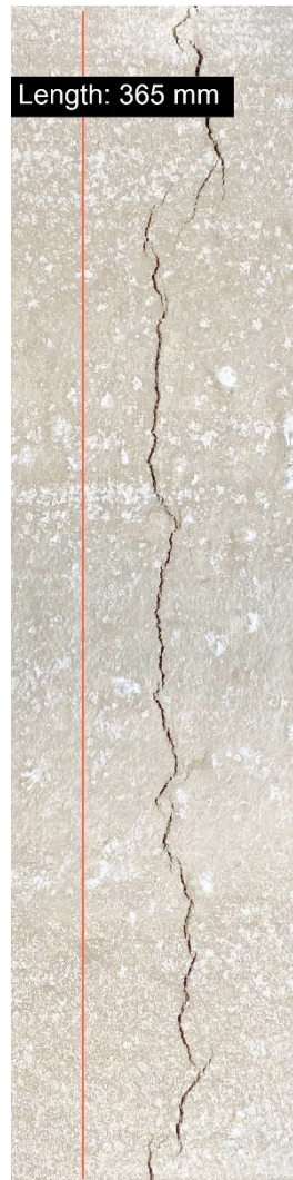
Figure C.37: IC crack length at 24 hours of plain concrete.
