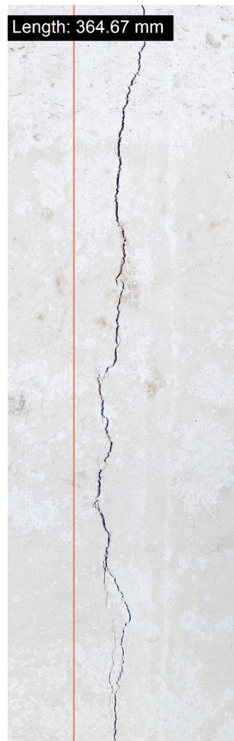
Figure B.29: IC crack length at 24 hours of plain concrete.
