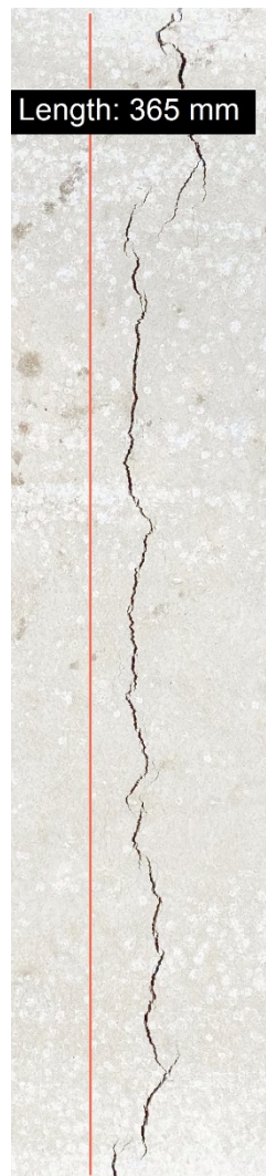
Figure C.16: IC crack length at 24 hours of plain concrete.
