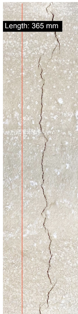
Figure C.22: IC crack length at 24 hours of plain concrete.
