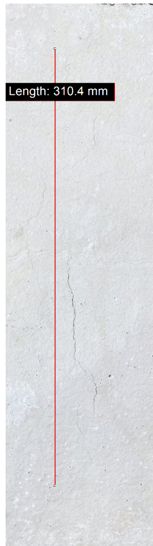
Figure B.32: IC crack length at 24 hours of MSFC30.
