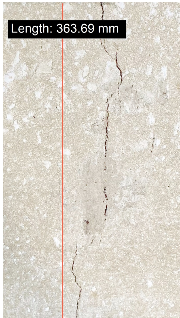
Figure C.1: IC crack length at 24 hours of plain concrete.
