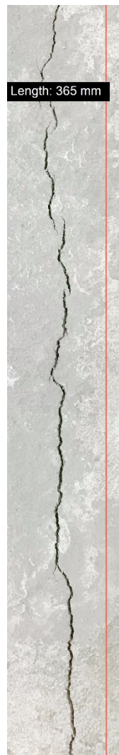
Figure C.40: IC crack length at 24 hours of plain concrete.
