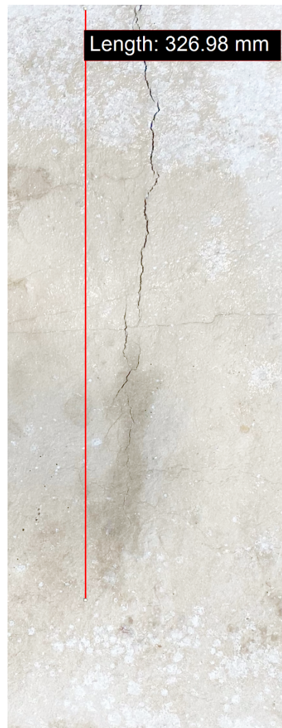
Figure B.23: IC crack length at 24 hours of plain concrete.
