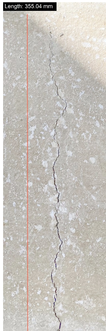
Figure D.28: IC crack length at 24 hours of plain concrete.
