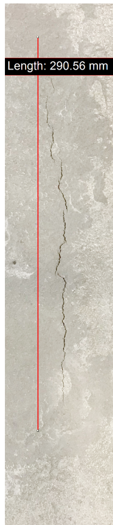
Figure B.26: IC crack length at 24 hours of MSFC20.
