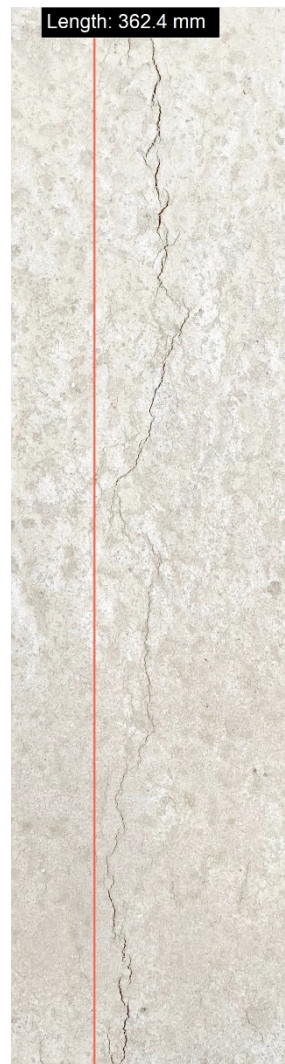
Figure D.31: IC crack length at 24 hours of SSC.
