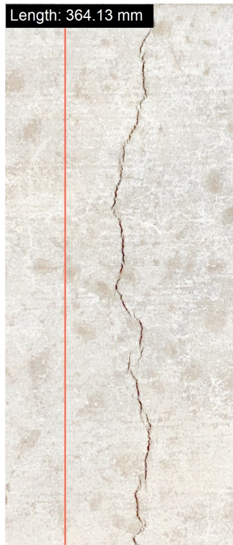
Figure D.34: IC crack length at 24 hours of plain concrete.
