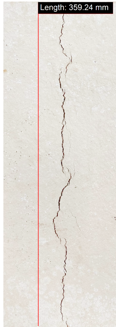
Figure B.17: IC crack length at 24 hours of plain concrete.
