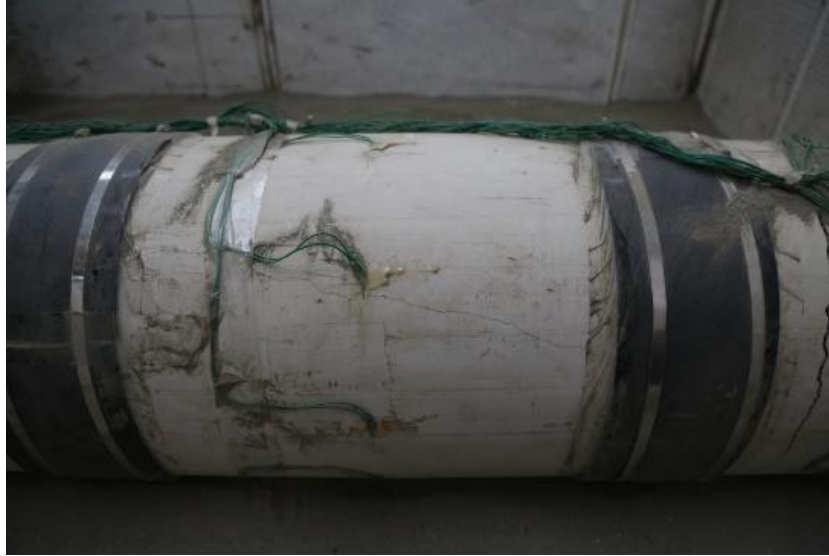
Figure 4.19: External damages of lining 3.
