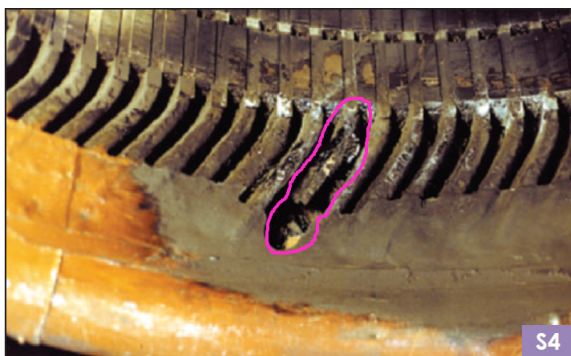
(c) A turn-to-turn short-circuit caused by a defective magnet wire insulation
