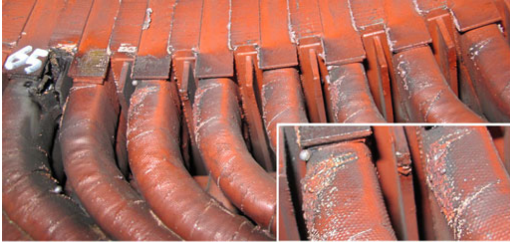
Fig. 1.18 Turn insulation failure in the end winding of a 6.6-kV, 1678-kW primary air fan motor [80].
