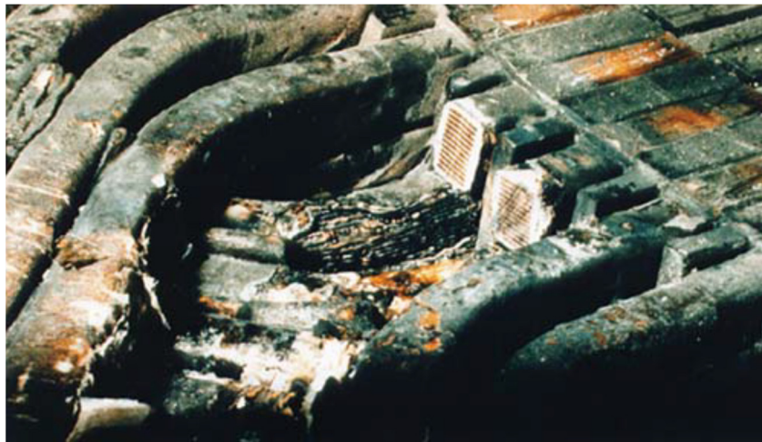
Fig. 1.17 A turn-to-turn short-circuit leading to a ground fault in a 6.6 kV, 8MW motor [78].
