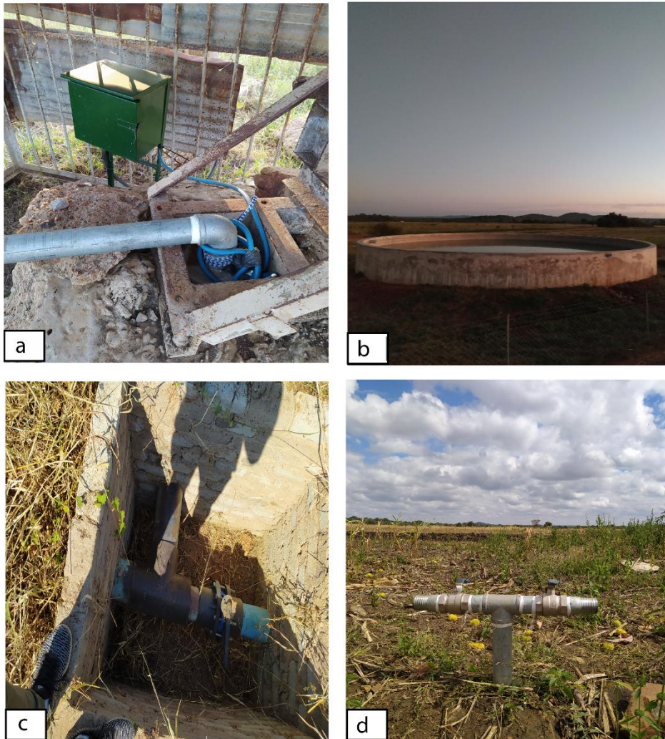
Figure 2. 5: a) Borehole equipped with submersible pump and mounted on a platform previously used for a mono pump; b) concrete tank which replaced the leaking earthen tank; c) a T-junction and gate valve for the control of water in the buried pipeline; and d) a hydrant fitted with a stop cock ball valve on which the pipes for irrigating the plots are connected. Source: Tavengwa Chitata (2020).
