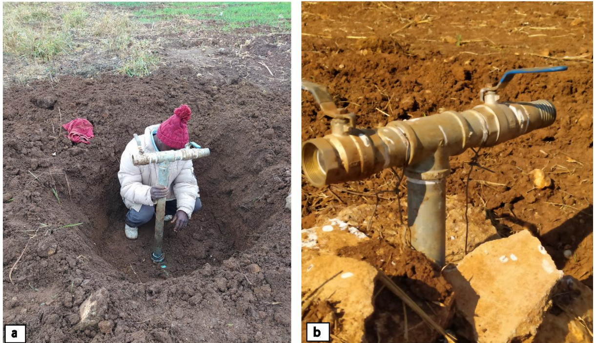
Figure 2. 7: a) Davison [an alias] assessing the plastic saddle-hydrant joint that was excavated to allow for repairs; b) hydrant fixed in position and made able to withstand water pressure, using a pair of wires tied on the T-wings and strapped to an underground pipe. Source: Tavengwa Chitata (2020).
