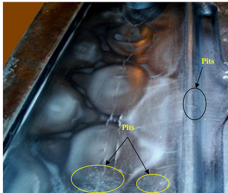
Figure 3.3 Illustration of erosive wear (picture was taken in Hallam Casting Company).
