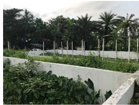
Figure 11: Lakshimpur Faecal Sludge Treatment Plant
