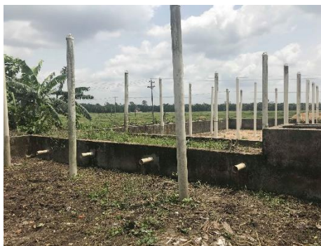
Figure 12: Chowmuhani Faecal Sludge Treatment Plant
