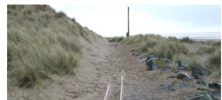
18: The track at Fairbourne showing the problems of construction the line on sand. A similar situation as Blackpool. (Source unknown.)
