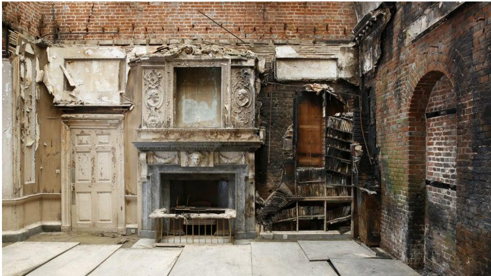
Figure 84 Clandon Park Library after the fire
