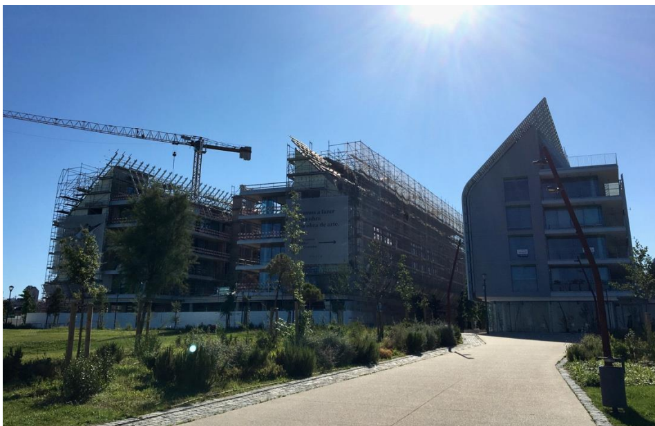
Figure 13: A section of VIC Properties' Prata Riverside Village, under construction. Photo by author.
