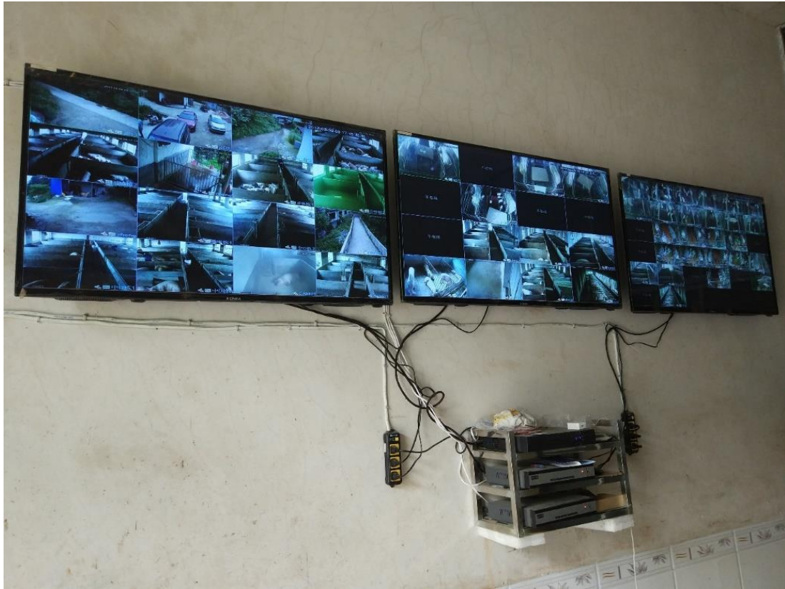
Figure 28 CCTV system in pig house
