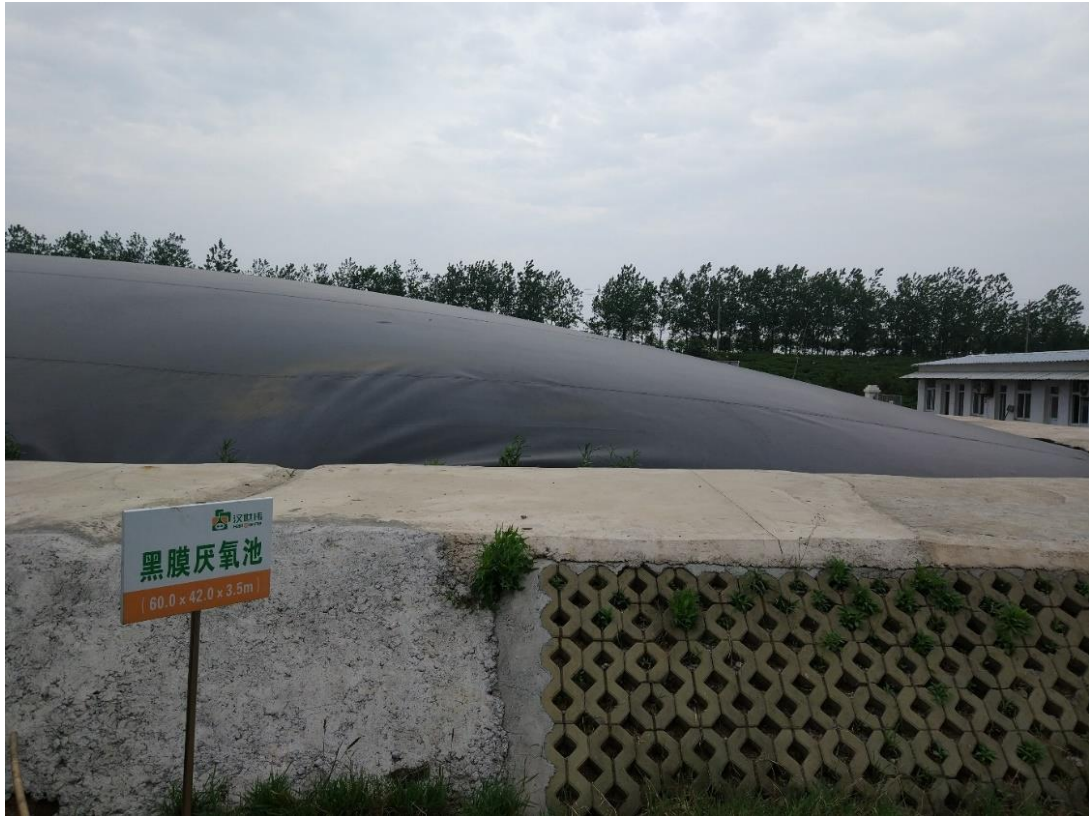
Figure 21 Anaerobic pool covered by black film
