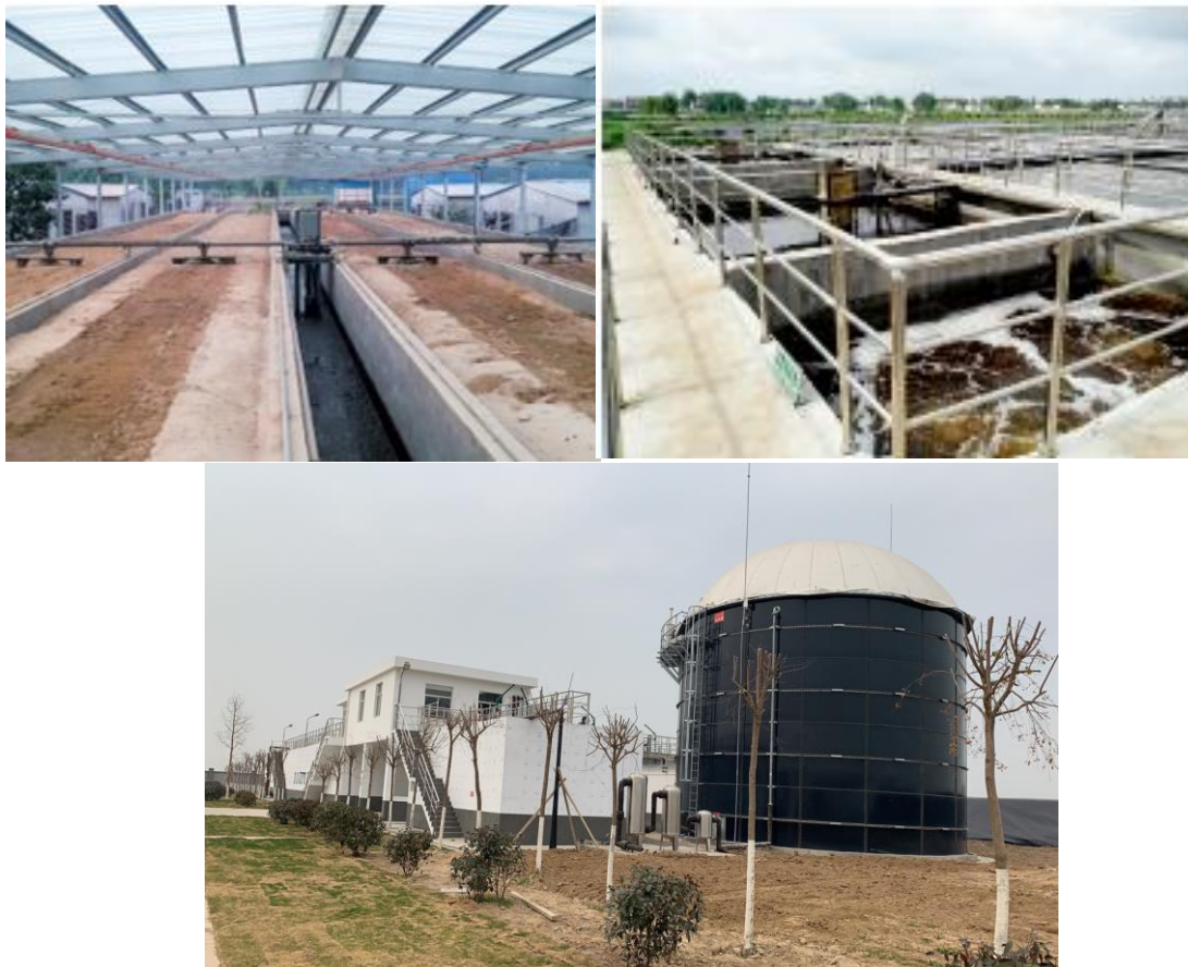
Figure 6.9 Lihua's pig farm sewage treatment facility
