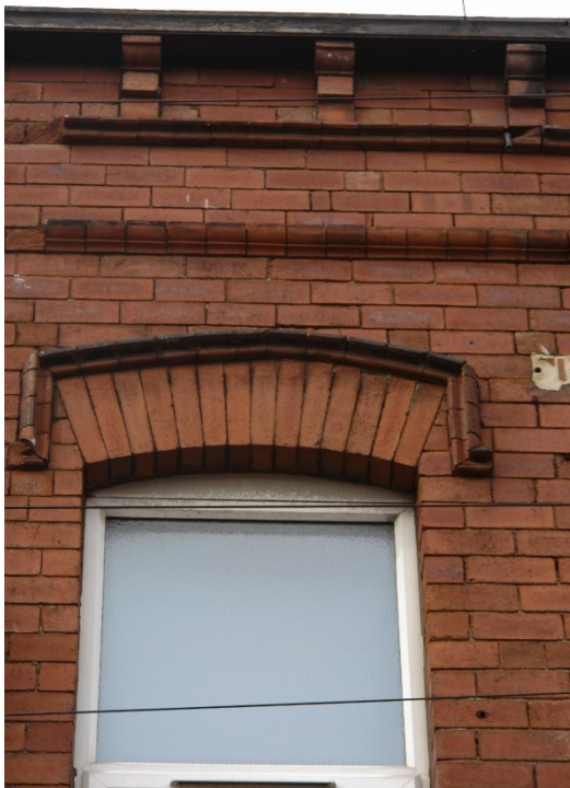
Figure 14 The gutter is supported off corbels, positioned above two decorative strings courses. A decorative string course flows across the façade, and over the top of the brick arched lintels.
