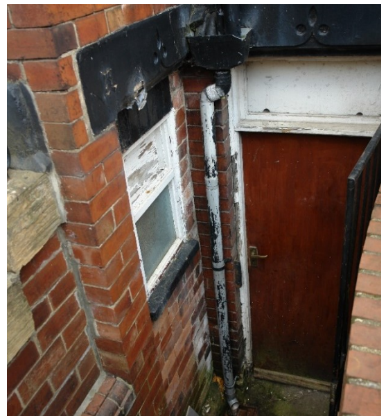
Figure 9 The original doorway to the toilet has been blocked up and had a window inserted in its place.
