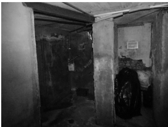
Figure 33 Large areas of the basement have been plastered with modern materials, directly onto the original brickwork - this has been problematic for the rooms as gypsum plaster should not be applied to solid walls, especially below ground level as it interferes with the breathability of the original fabric. A small amount of original brick flooring remains in the small room to the left of the bottom photo.
