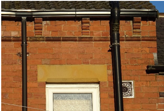
Figure 8 The gutter is supported off corbels, positioned above a plain string course. The plain stone reflects the plainer Edwardian style. The original decorative air brick can be seen next to the window.
