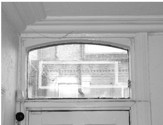
Figure 20 The arch top fanlight - the frame is original but the glass has been replaced.
