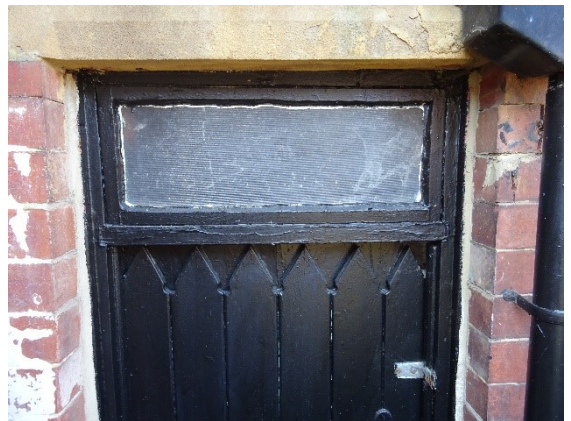
Figure 11 The original toilet door remains, but the ventilation gap at the top has been blocked with timber.
