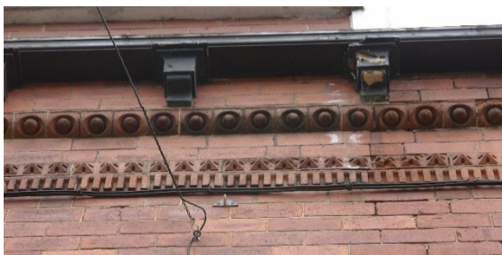
Figure 17 The timber gutter is supported by stone corbels positioned above a decorative frieze comprising three separate string course designs.
