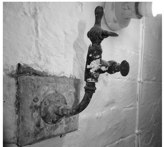
Figure 25 Gas light valve.
