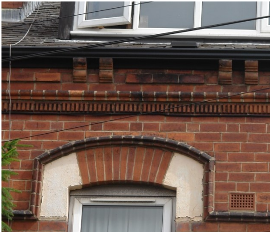
Figure 14 The timber gutter is supported on double brick corbels with a decorative brick frieze between and below.
