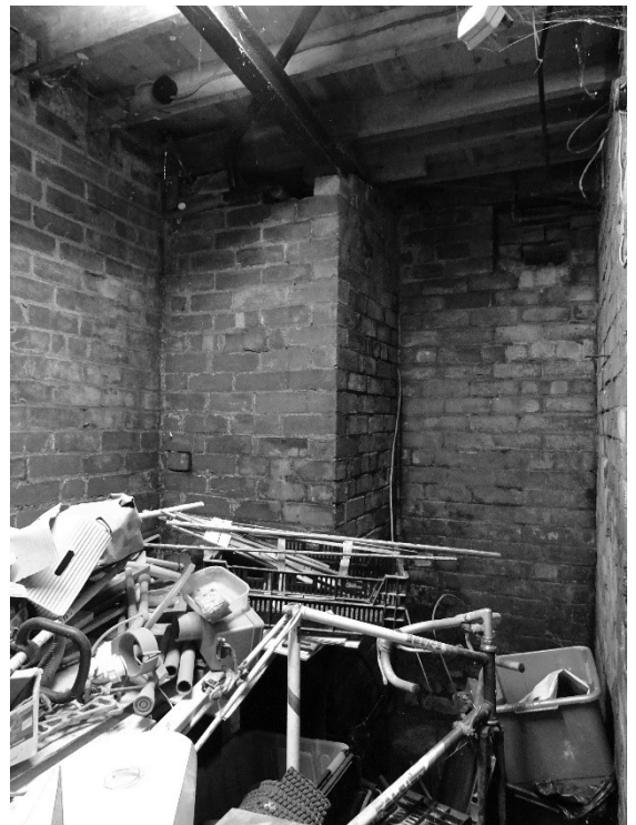
Figure 31 The small basement room has had the lath and plaster ceiling removed and has been strengthened with steel. This was likely done during the war and would have had a corrugated steel sheet underdrawing.
