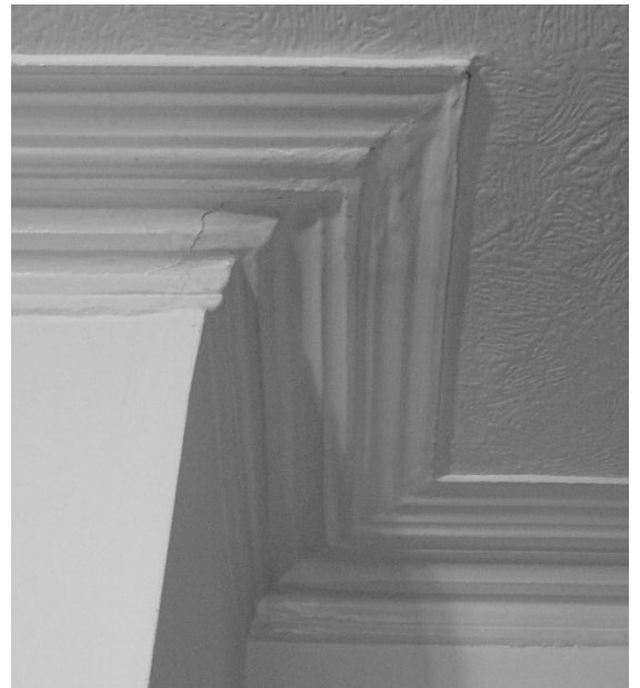
Figure 21 The original cornice in the living room, damaged in places.
