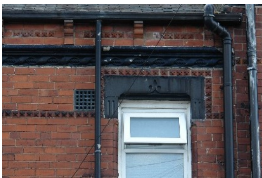
Figure 6 The gutter is supported off corbels, positioned above a decorative stone string course. A decorative brick string course flows across the façade, and over the top of the decorative stone lintels.
