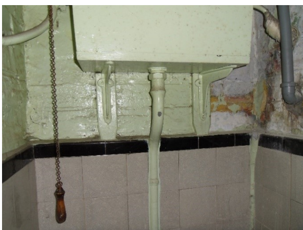
Figure 272 High level cistern and wall tiling to a WC that is accessible both internally and externally.
