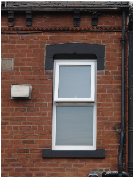
Figure 16 The gutter is supported off corbels, positioned above two decorative strings courses. The decorative lintel and sill are characteristic of the area.
