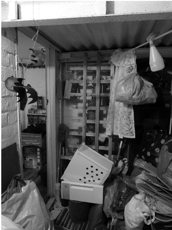
Figure 20 The small basement room was strengthened during war time, as evidenced by the steel beam and corrugated steel sheet underdrawing to the floorboards above.
