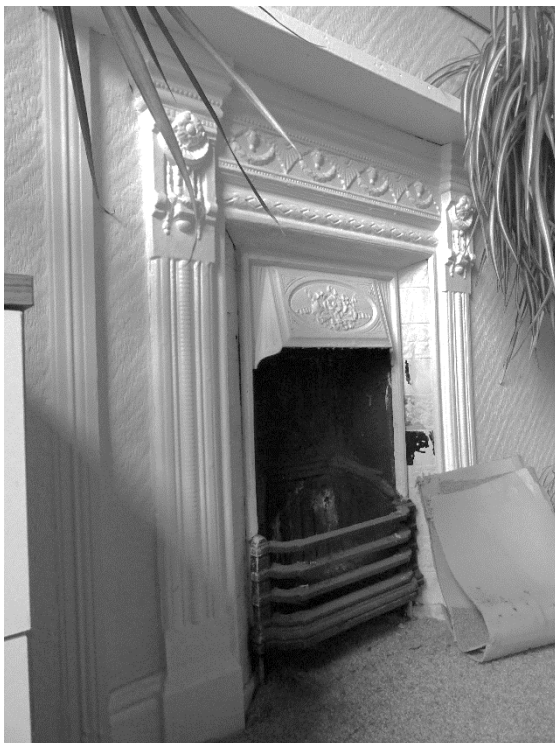
Figure 30 The original cast iron fireplace to the bedroom is very ornate and in good condition.
