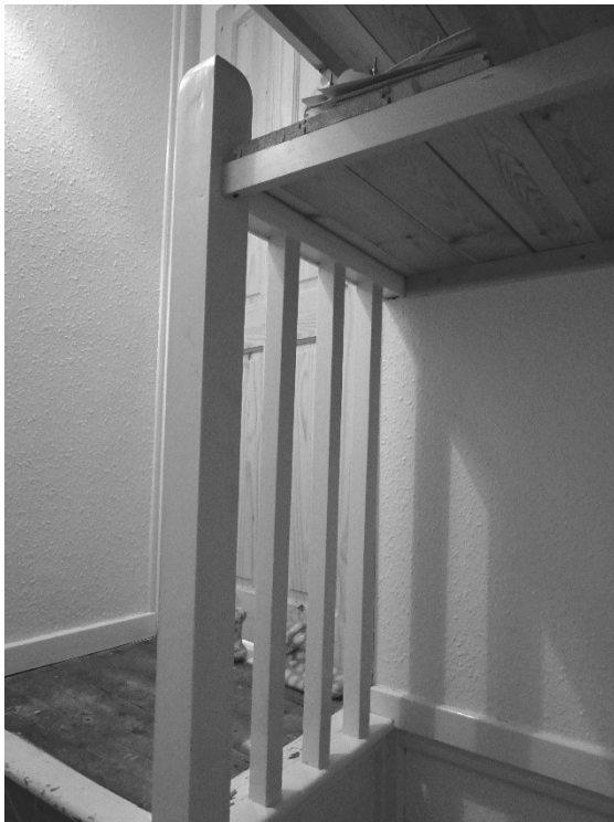
Figure 29 Original balustrade and newel post to the attic floor (originally open to the attic space).
