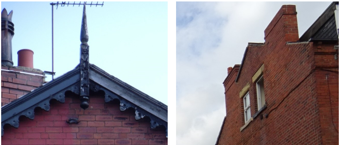
Figure 12 Gable post with decorative bargeboards featuring a scalloped edge and perforations (left); and mortar-bedded verge (right).
