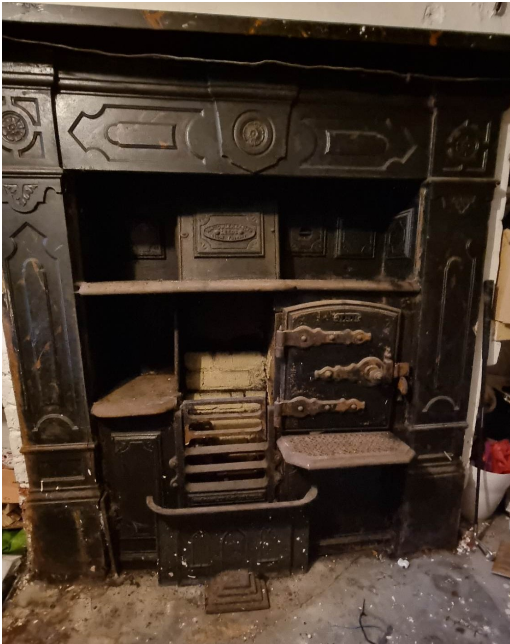
Figure 22 An extant range in a basement room, complete with ovens, pan stands, grates and mantel (Korotkevic 2022).
