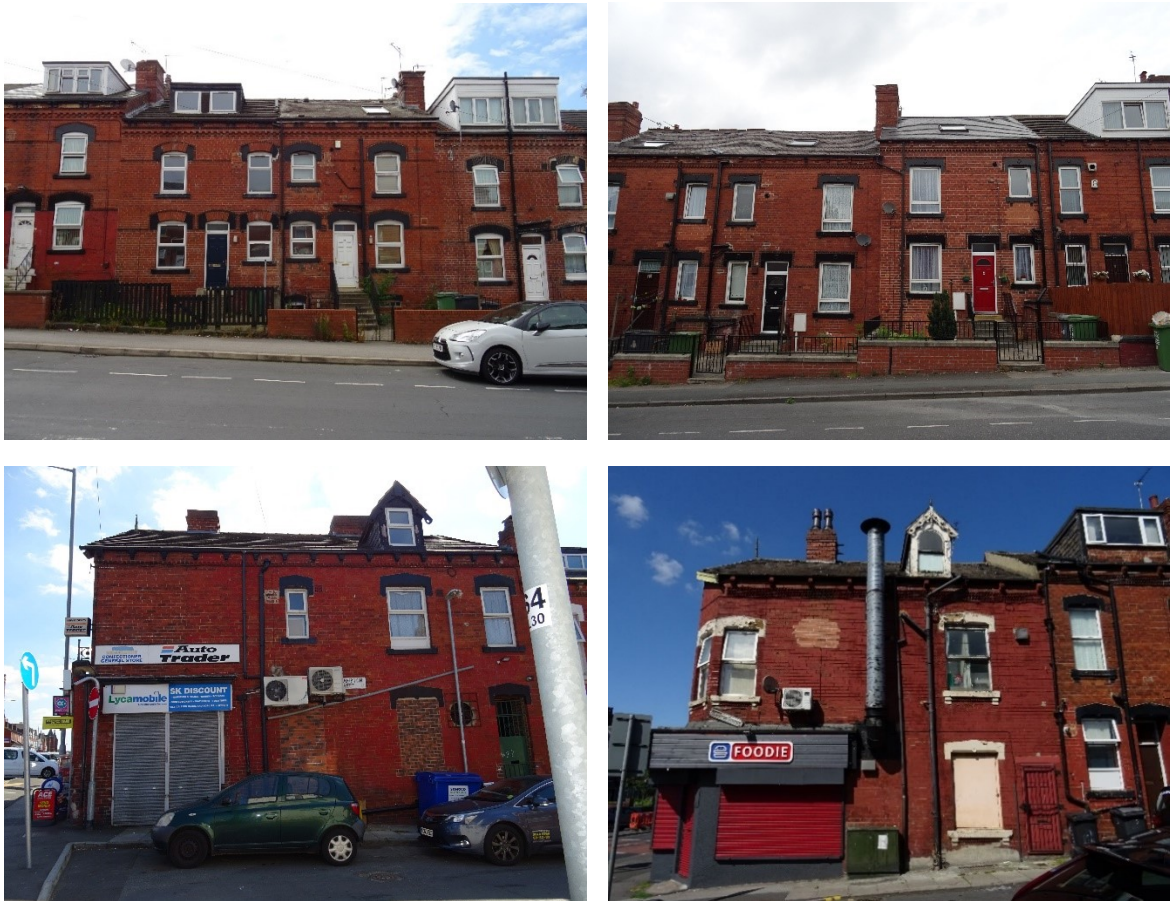
Figure 34 Raised windowsills (top); bricked up window and door (bottom left); boarded window (bottom right). All impact negatively on the streetscape because they disrupt the rhythm of the fenestration.
